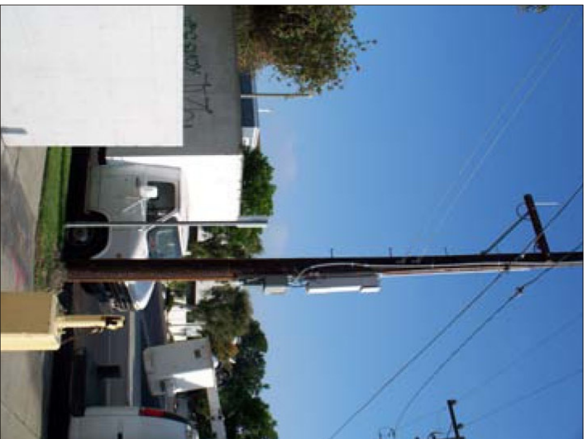
Photo 2: Typical Node Installation
