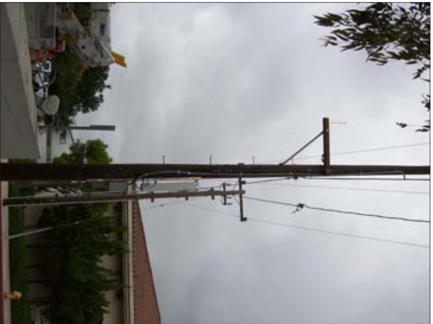
Photo 1: Typical Node Installation
