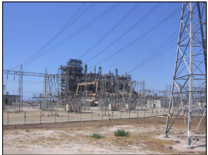
Photo 2: View of South Bay Substation Looking South
