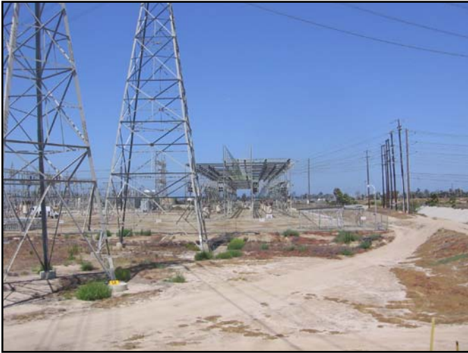
Photo 1: View of South Bay Substation Looking West
