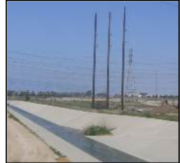
Three-pole wood riser structure
