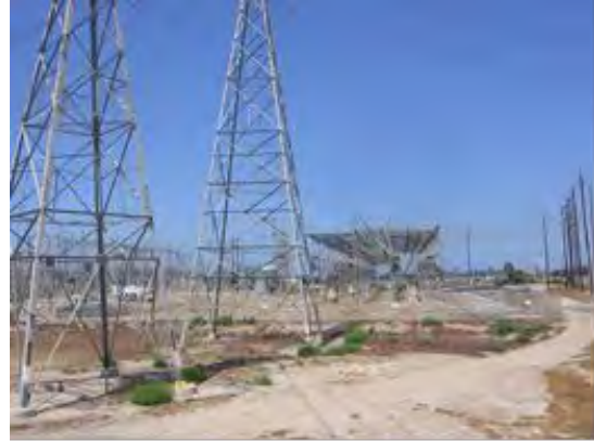
Photo 2: Looking west at the South Bay Substation (to be dismantled)
