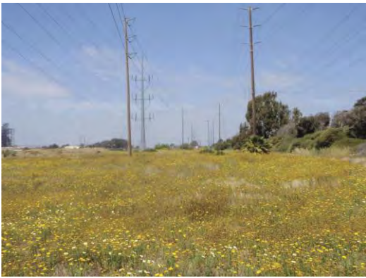
Photo 3: View of the ROW east of the proposed Bay Boulevard Substation, looking north
