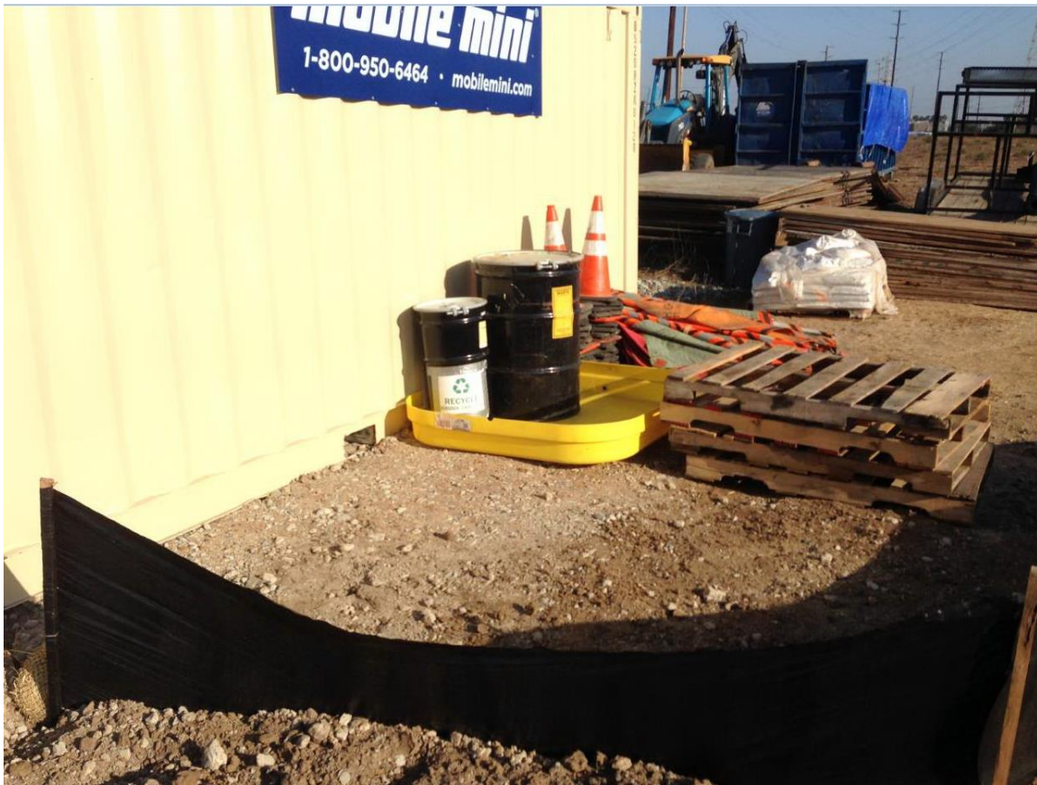
Photo 6: Equipment including dumpsters, heavy vehicular equipment, building materials, etc. was staged along the transmission line alignment. Silt fencing was installed around staging areas, waste bins were observed contained, absorbent material was observed under staged vehicular equipment, and dumpsters were observed covered and secured to prevent attracting wildlife.
