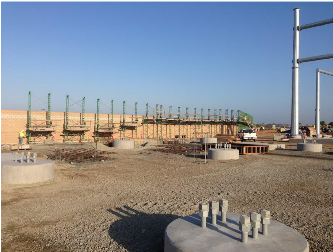
Photo 3: Masonry work on the construction screening wall (above) and control shelter continued this reporting period. Vertical components of the Bay Boulevard Substation (structural steel, above, right) was observed being erected by equipment.
