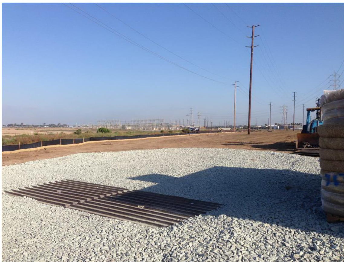
Photo 5: After work limits were delineated along the transmission alignment, SWPPP BMPs were installed, including silt fencing, straw wattles, and a stabilized construction entrance consisting of a rock apron and rattle plates.
