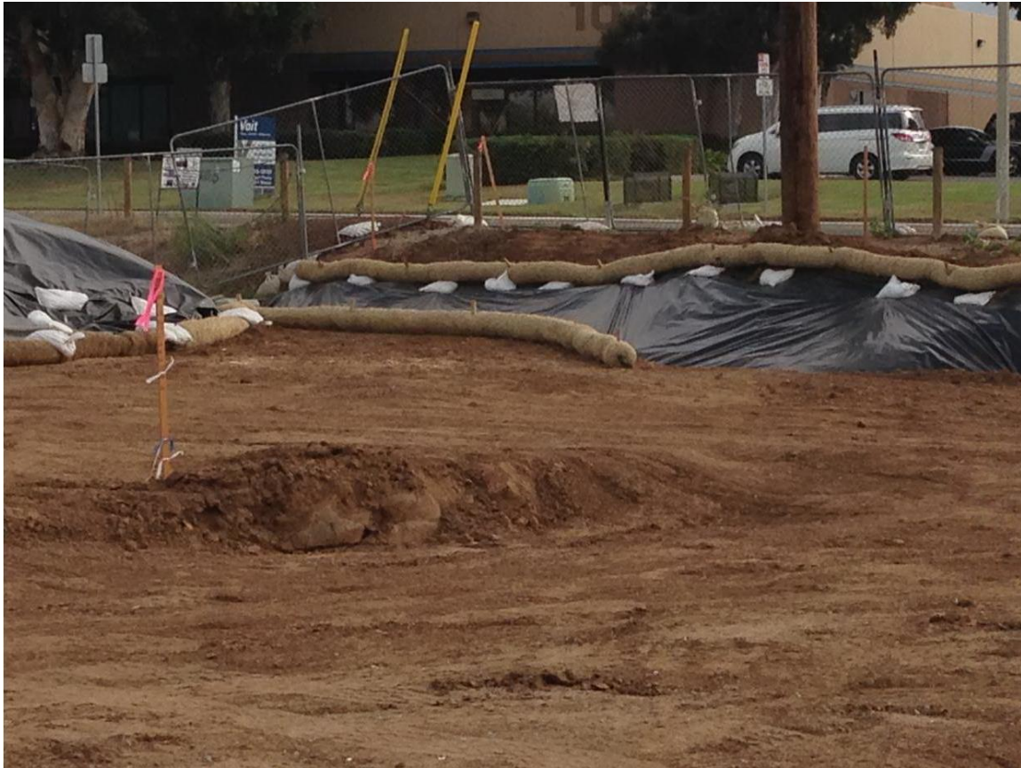
Photo 1: Prior to an anticipated rain event, visqueen secured by gravel bags and straw wattles were observed along the Bay Boulevard Substation box culvert/southern driveway in accordance with the SWPPP. Stockpiles were also secured with visqueen, gravel bags, and straw wattles prior to the event, and runoff was not reported.
