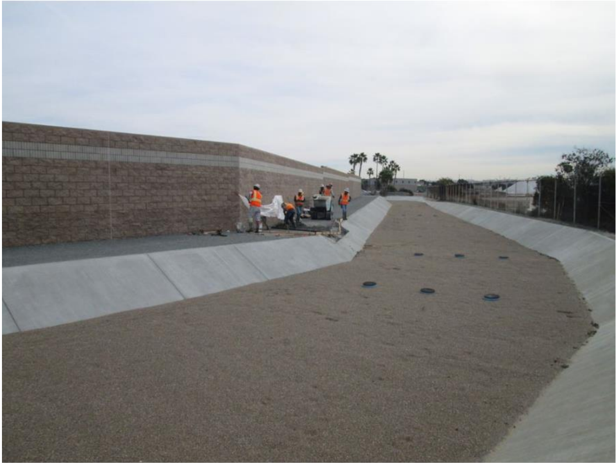
Photo 1: Crews were observed placing concrete forms in the Bay Boulevard Substation screening wall outlets.
