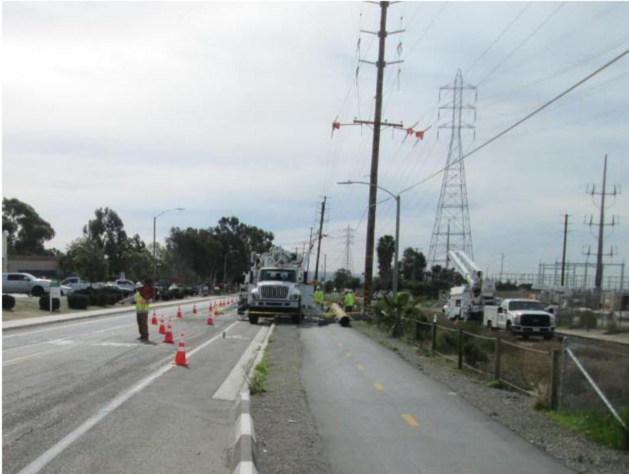
Photo 6: Crews were observed preparing a new 69kV pole for installation along Bay Boulevard. Traffic control flaggers were used to divert traffic around staged equipment in accordance with MM TRA-1.
