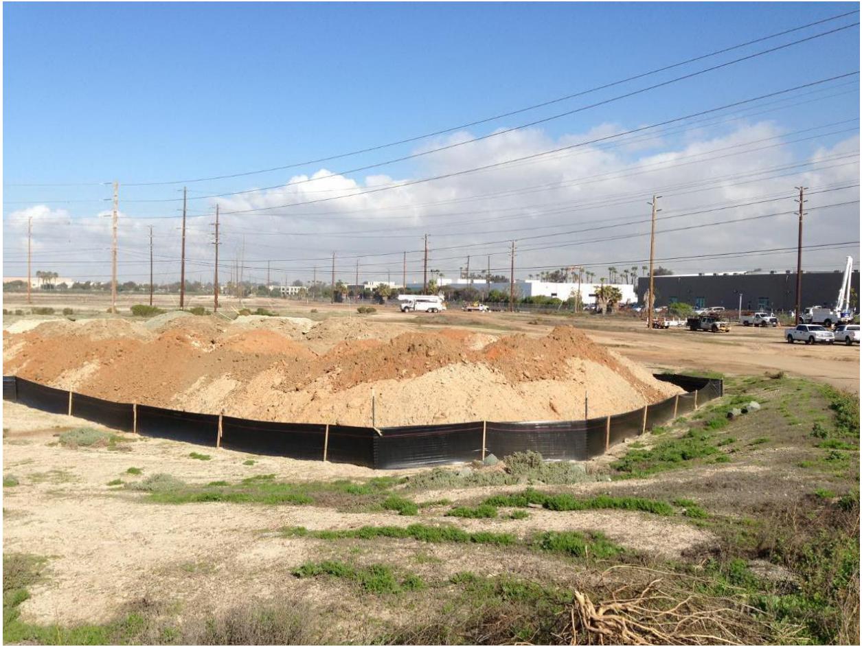
Photo 4: Stockpiles along the transmission line alignment were secured with silt fencing in accordance with the SWPPP.
