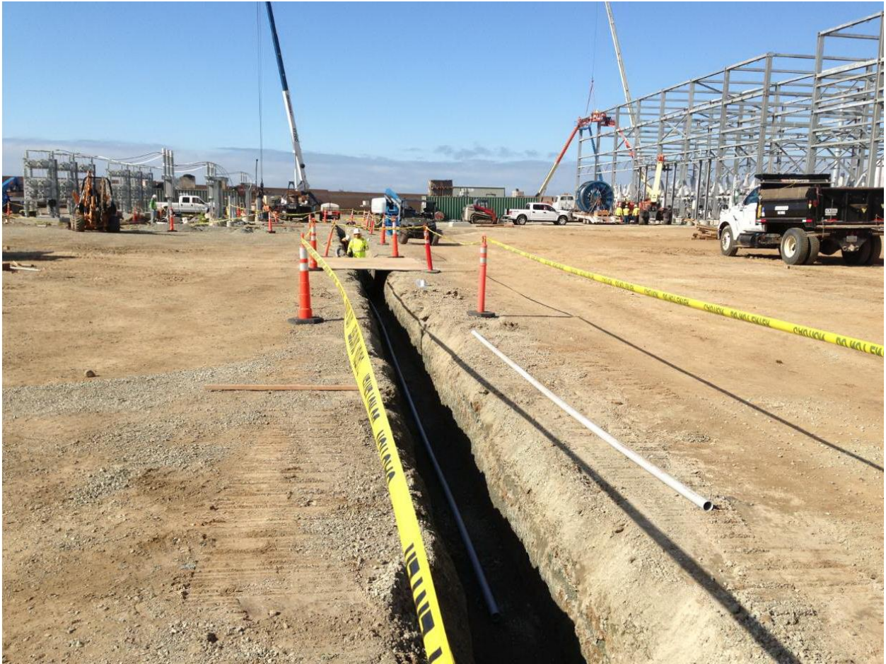
Photo 2: Crews were observed erecting steel at the Bay Boulevard Substation and continuing to install conduit.
