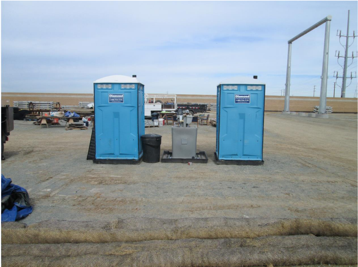
Photo 5: Portable sanitation facilities (i.e. toilets and wash stations) were observed on catchment units in accordance with SWPPP.
