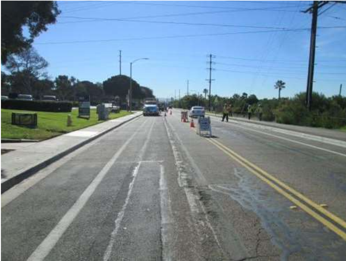
Photo 2: During potholing activities along Bay Boulevard, crews were observed implementing traffic control measures in accordance with MM TRA-1 and the Traffic Control Plan.
