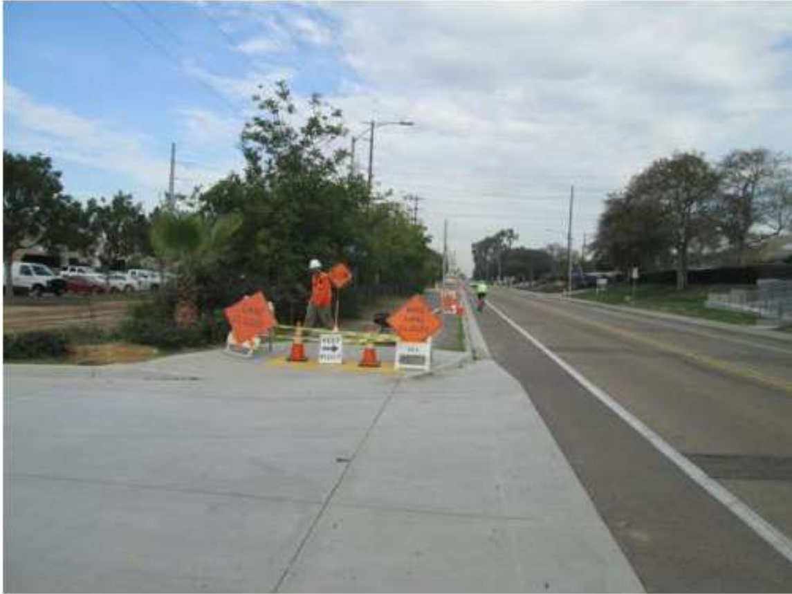
Photo 3: During potholing activities within the Bay Boulevard bike path, traffic control personnel and detour signs were located on both sides of the construction area to direct bicyclists to an alternate route in accordance with MM TRA-5.
