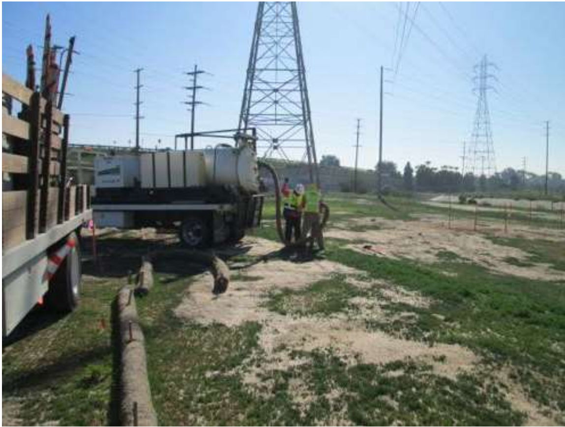
Photo 4: Potholing activities were conducted within the Bay Boulevard substation footprint. Crews were observed working with straw wattles installed around equipment and drip pans were observed placed under vehicles to contain any potential leaks accordance with the project SWPPP.
