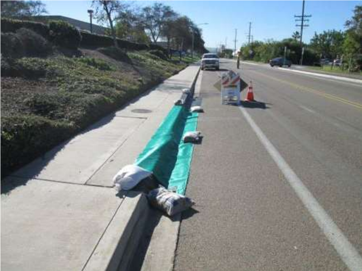
Photo 1 Prior to initiating potholing activities, crews were observed placing sediment control devices (consisting of filter fabric and gravel bags) around the storm drain inlets in accordance with MM HYDRO-1 and BMP 1-06 of the project SWPPP.
