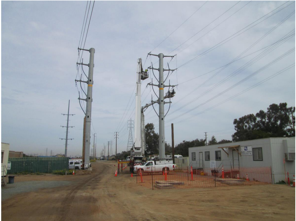
Photo 1: Crews were observed sagging 69kV wire along a transmission line within the right-of-way.
