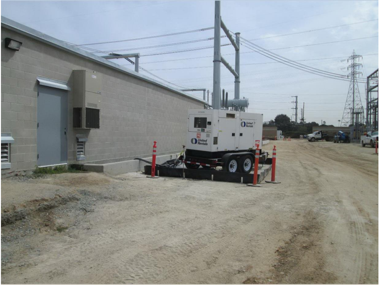
Photo 4: Generators were stored within catchment areas to prevent potential contamination of soil in accordance with project SWPPP BMPs (MM HYDRO-1).
