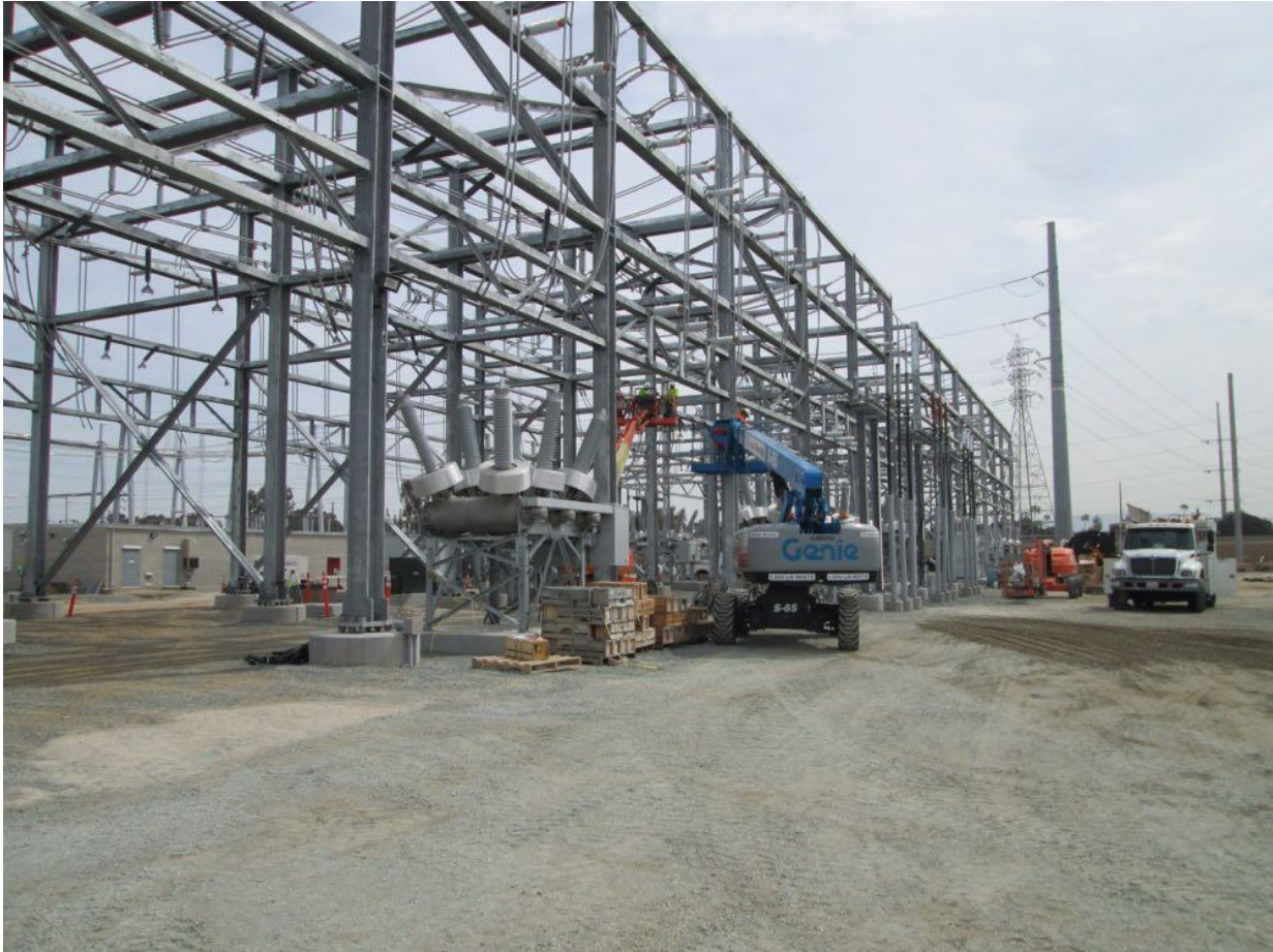
Photo 2: Crews were observed conducting wire termination work at the 69kV rack at the Bay Boulevard Substation. Installation of bird deterrents/ribbons were reported to be installed within the racks by SDG&E on April 22, 2016.
