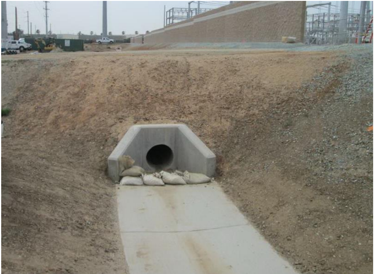
Photo 3: Gravel bag berms were observed placed along drainage channel inlets in accordance with the project SWPPP BMPs (MM HYDRO-1).
