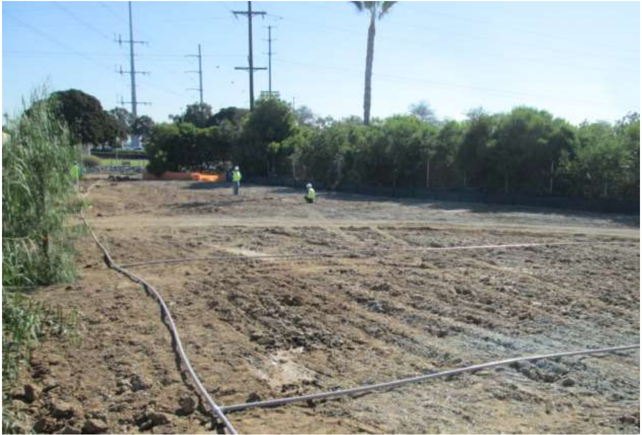
Photo 1: Crews were observed installing irrigation systems to support landscape planting adjacent to the Bay Boulevard Substation in accordance with the Conceptual Landscape Plan (APM AES-01).
