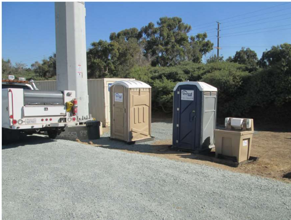
Photo 4: Containment was observed underneath wash stations and portable sanitation facilities in accordance with the project SWPPP (MM-HYDRO-01).
