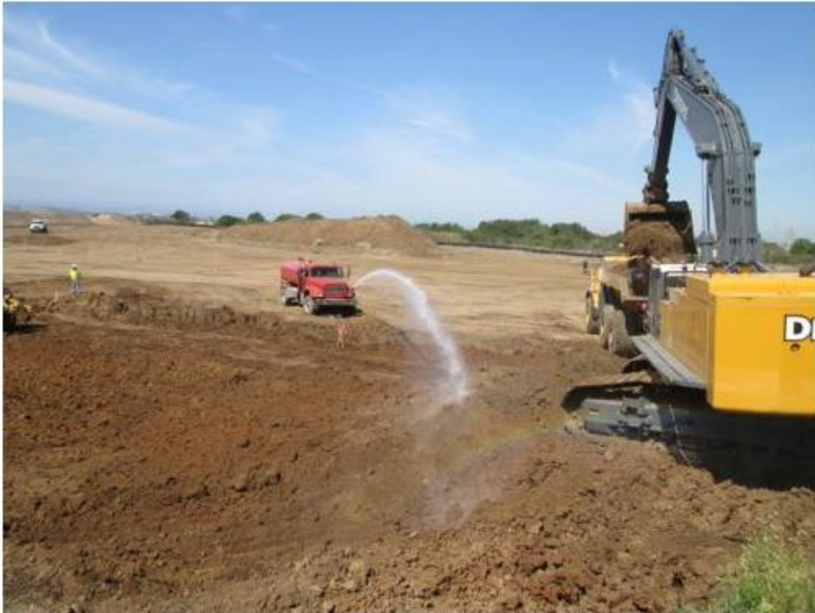
Photo 2: A water truck was observed being utilized to water excavation areas in order to minimize dust emissions in accordance with APM AIR-01.
