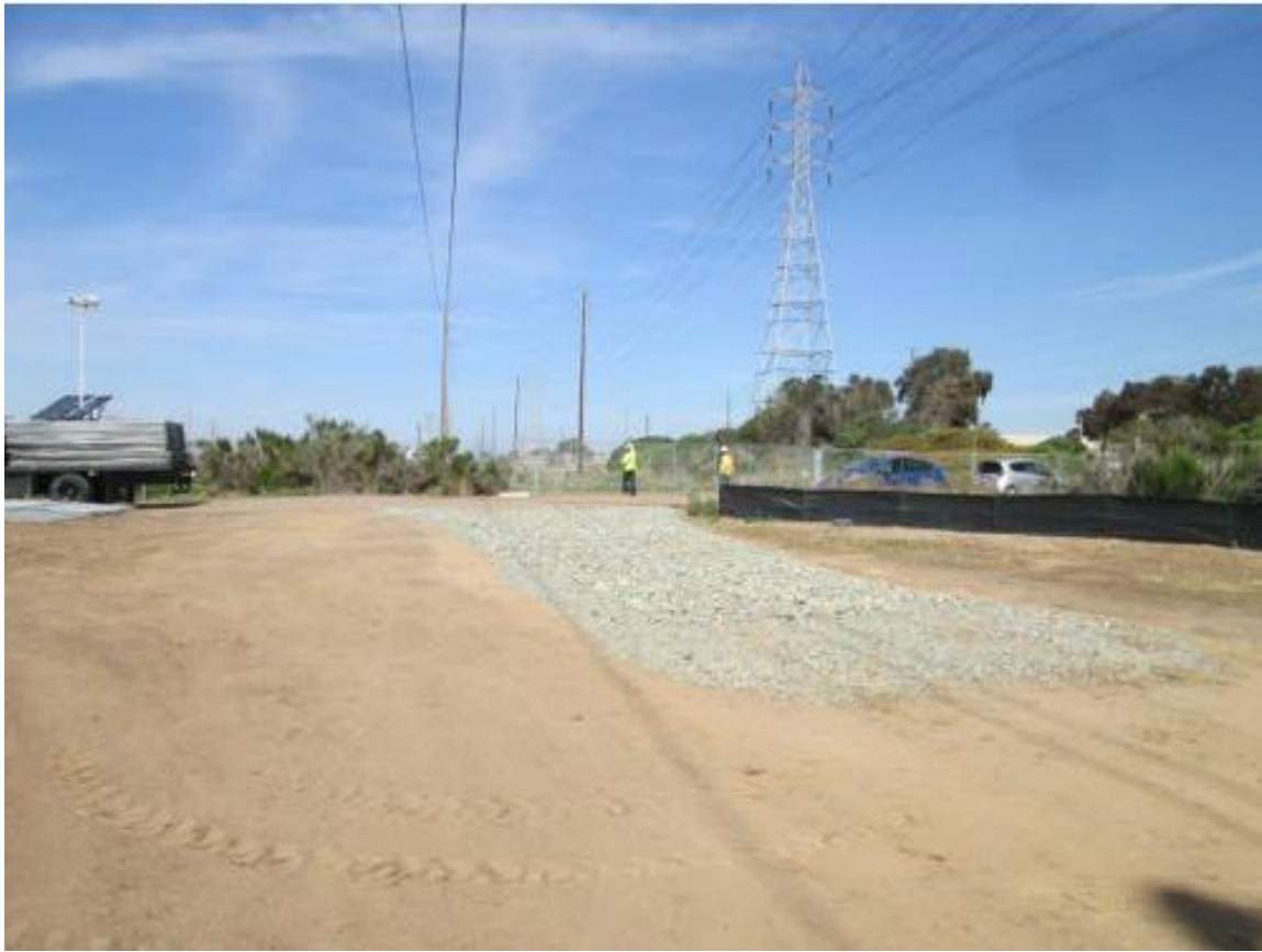
Photo 4: Installed rock aprons at the point of ingress and egress to minimize dirt/mud tracking from the site onto paved roads were observed in good condition in accordance with MM HYDRO-1.
