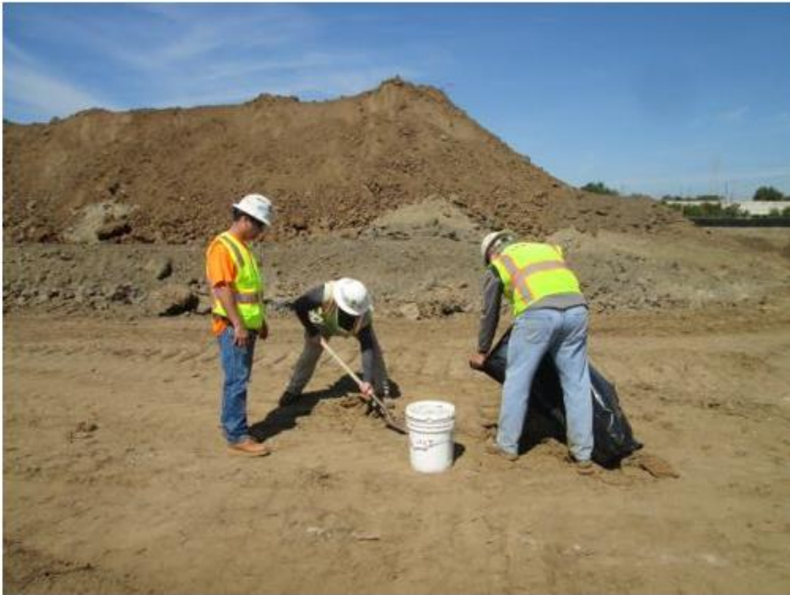
Photo 6: Crews were observed cleaning and containing stained soils on the project site in accordance with APM HAZ-01.
