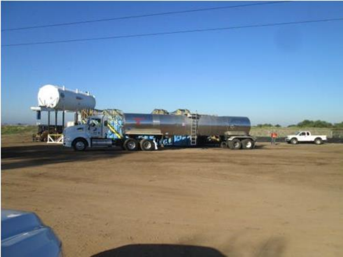
Photo 3: Baker tanks were observed on site to store reclaimed water for dust control and soil compaction during construction.
