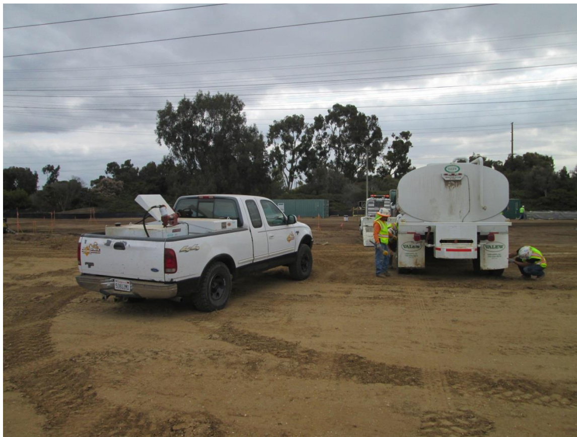
Photo 4: Crews were observed cleaning mud from a water truck prior to hauling offsite to prevent sediment track-out from the project in accordance with the project SWPPP and to reduce potential for offsite transport of weedy material in accordance with MM BIO-4.
