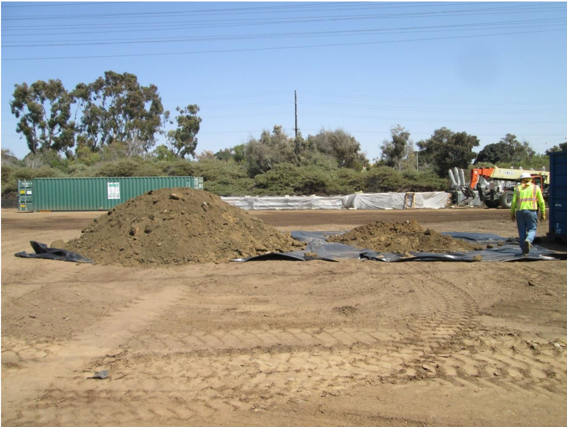
Photo 6: Excavated soil containing buried trash was observed temporarily stockpiled on visqueen for future disposal in accordance with APM BIO-01.
