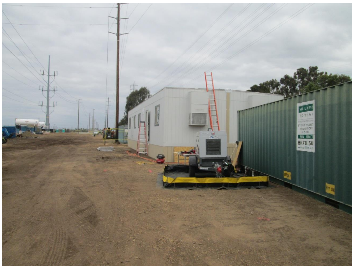
Photo 5: Spill containment was observed under equipment such as the generator used to service the temporary construction trailer in accordance with APM HAZ-1.
