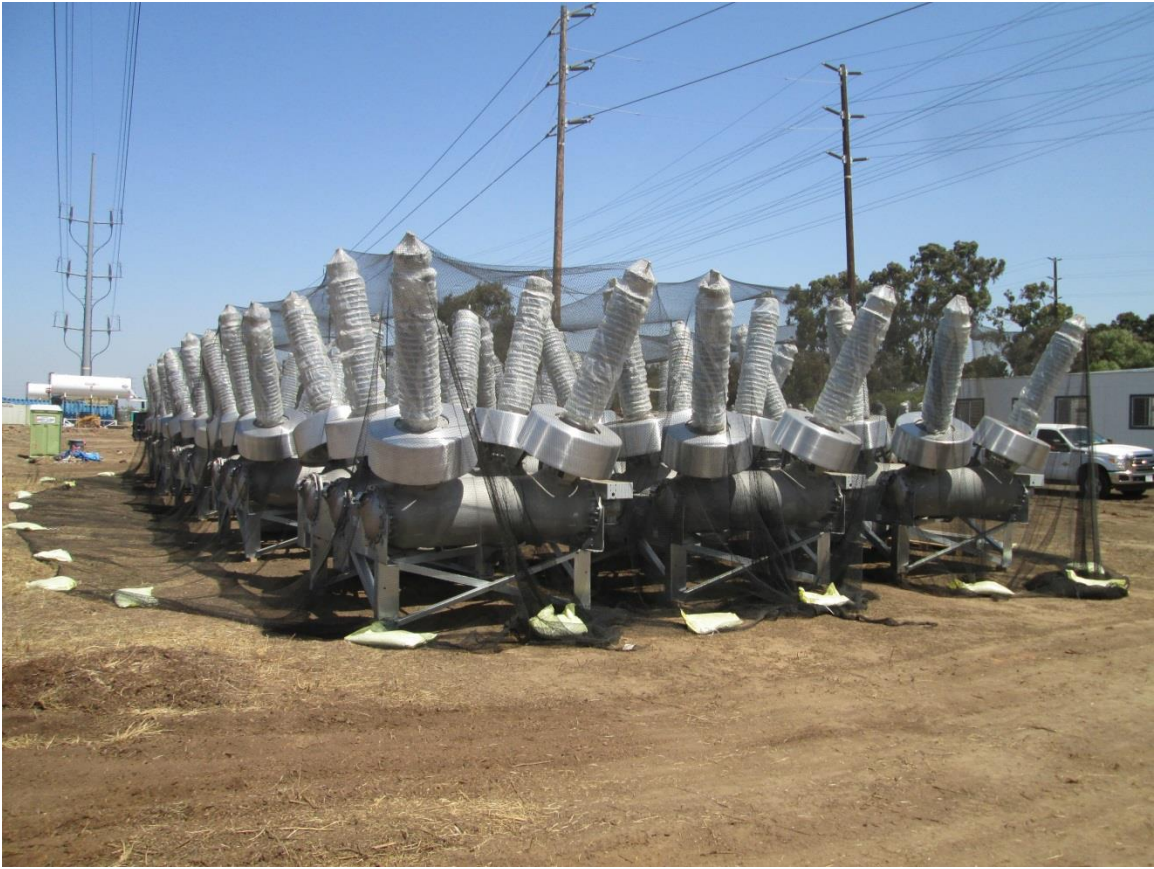
Photo 2: Netting material were placed over staged project equipment, such as circuit breakers and transformers, to deter birds from nesting in equipment.
