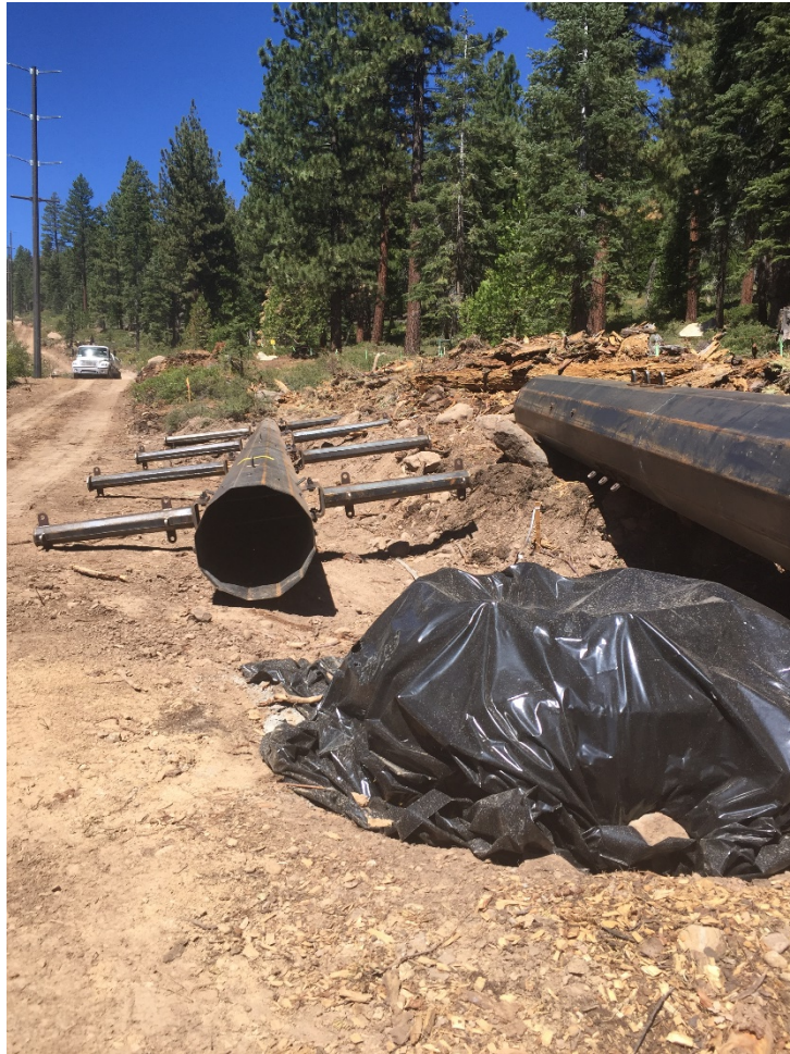
Photo 1: Pole top and bottom staged in ROW, poured concrete pole base covered. Approved work area flagged (APM-BIO-26).
