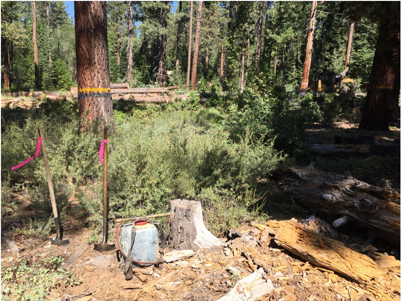
Photo 5: Firefighting equipment on site for timber operations, in accordance with APM-HAZ-6.
