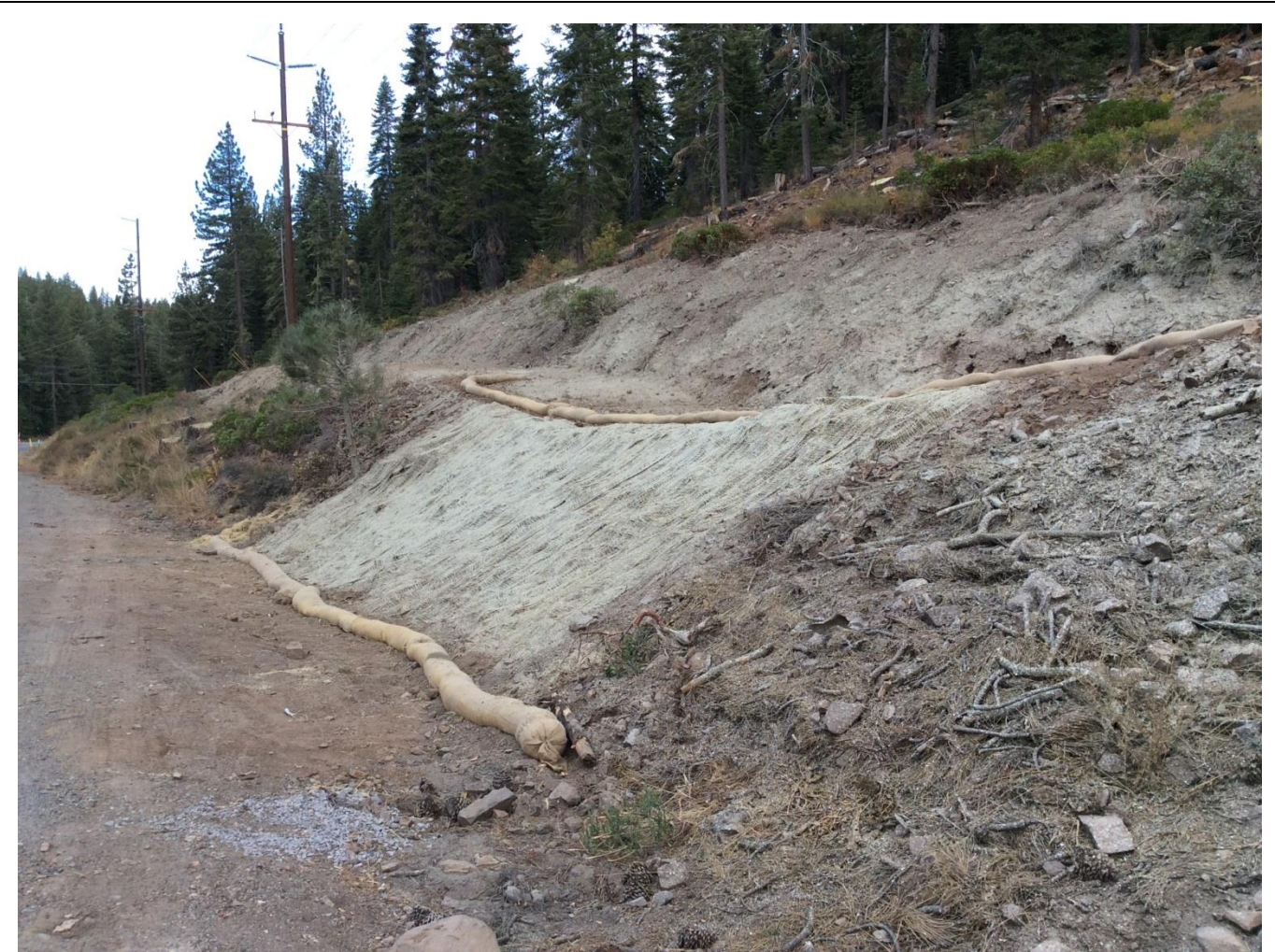
Photo 3: Temporary right-of-way access point re-graded with erosion control fabric, wattles, and hydroseed installed.
