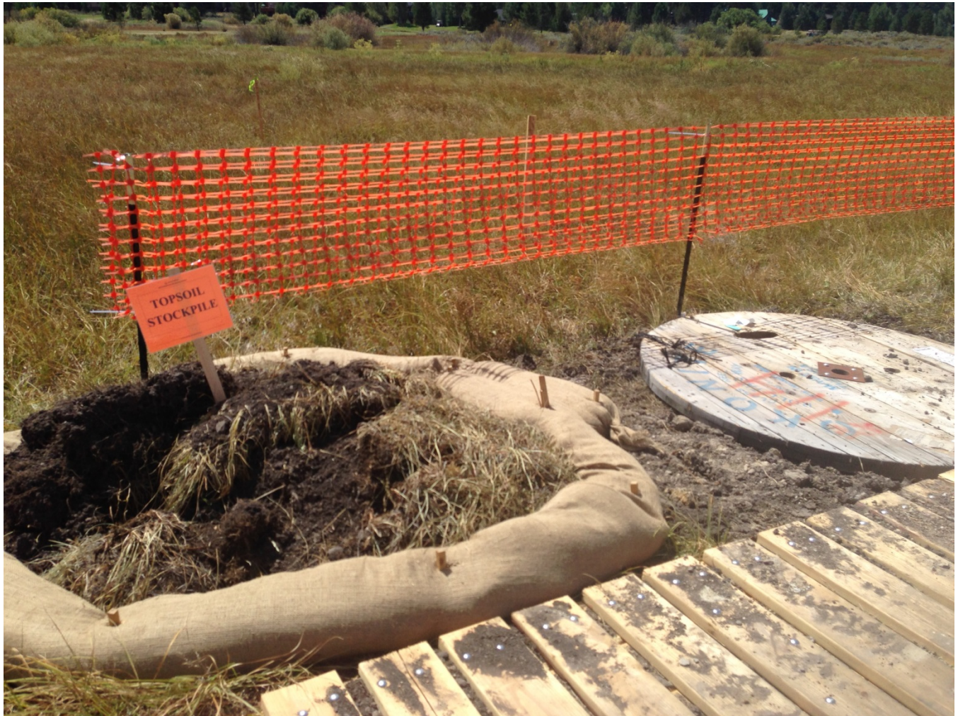
Photo 5: Topsoil salvaged and segregated in accordance with APM-BIO-23; however, the pile is not covered, as required under APM-BIO-23. Liberty Utilities stated they will cover topsoil piles, which will be confirmed in subsequent compliance inspections.
