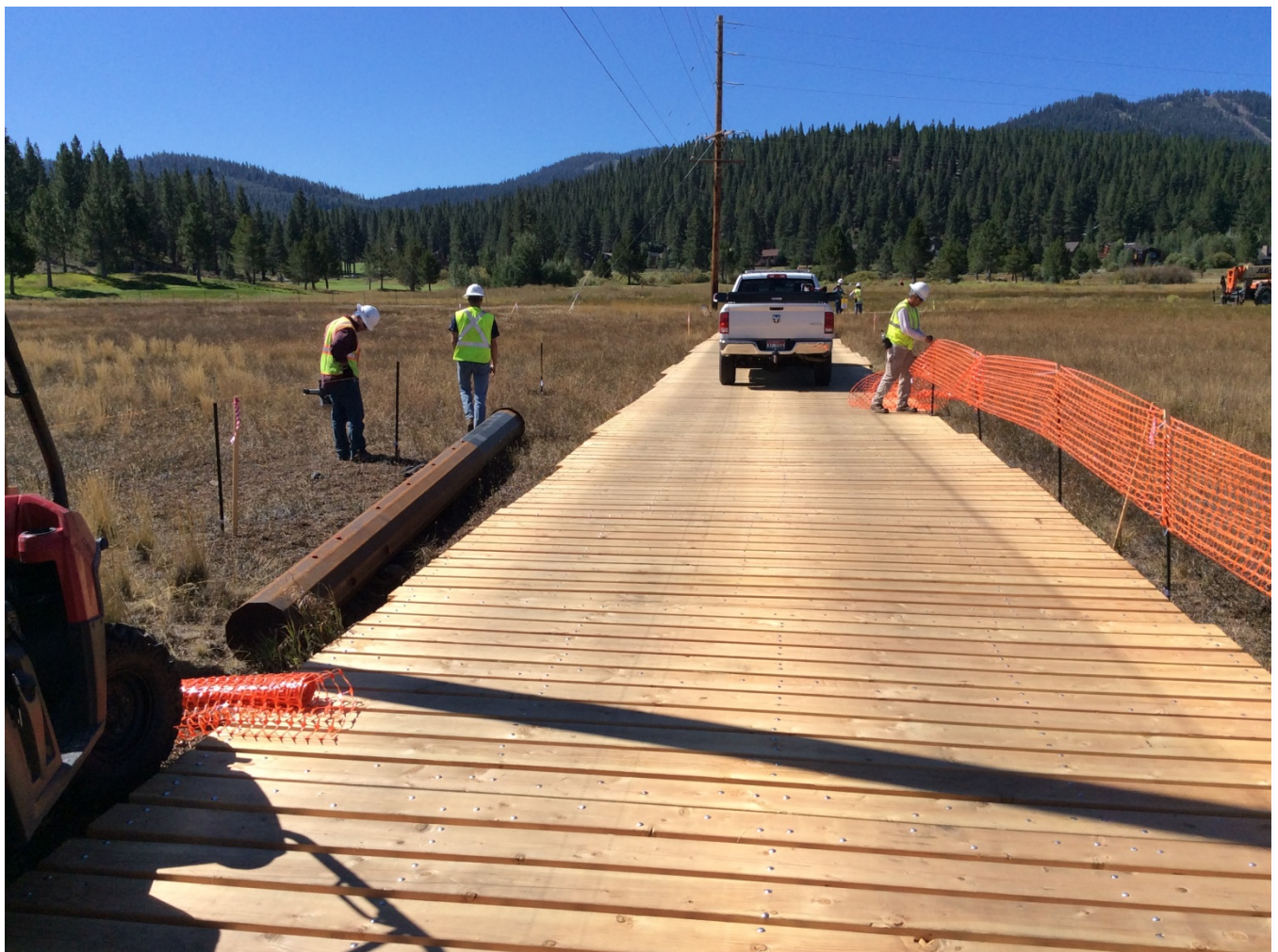
Photo 1: Crews installing work area fencing in Martis Valley to delineate approved work areas, consistent with APM-BIO-26 and the project's Flagging, Fencing, and Signage Plan. Work in this area is restricted to a 20-foot-wide portion of the ROW and timber matting has been installed to minimize impacts from vehicle and equipment travel. Also note that clearance is being provided at fence bottoms to allow for wildlife movement through the ROW.
