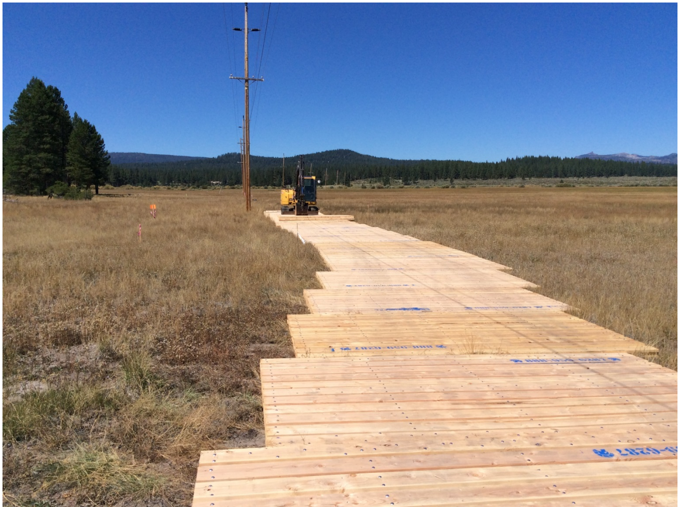
Photo 2: Timber matting being installed within the 20-foot-wide portion of the ROW to minimize impacts from vehicle and equipment travel
