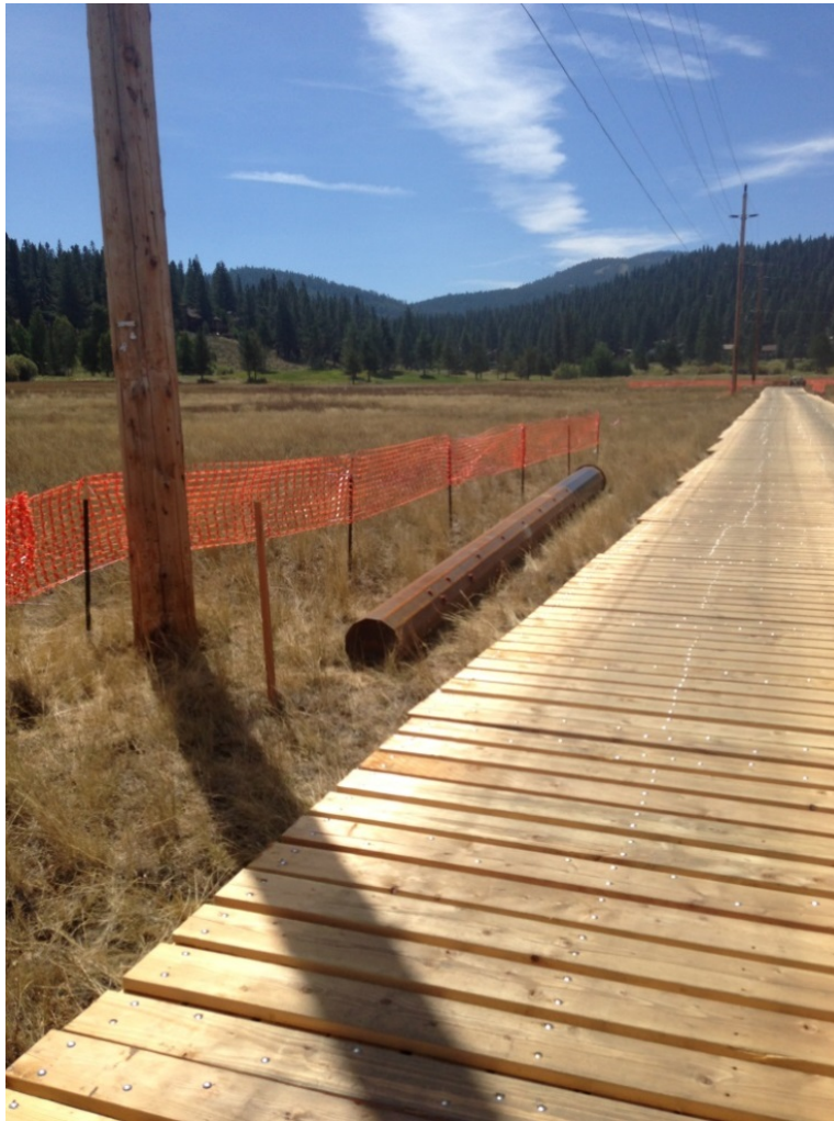
Photo 6: Material being staged inside fenced work area with project access via timber matting through Martis Valley.
