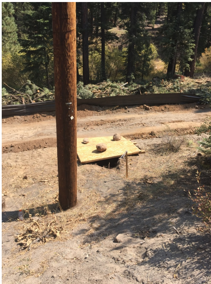
Photo 3: Ineffective covering of excavated pole hole. Monitors to inspect excavated pole holes daily for trapped wildlife, consistent with APM-BIO-22.
