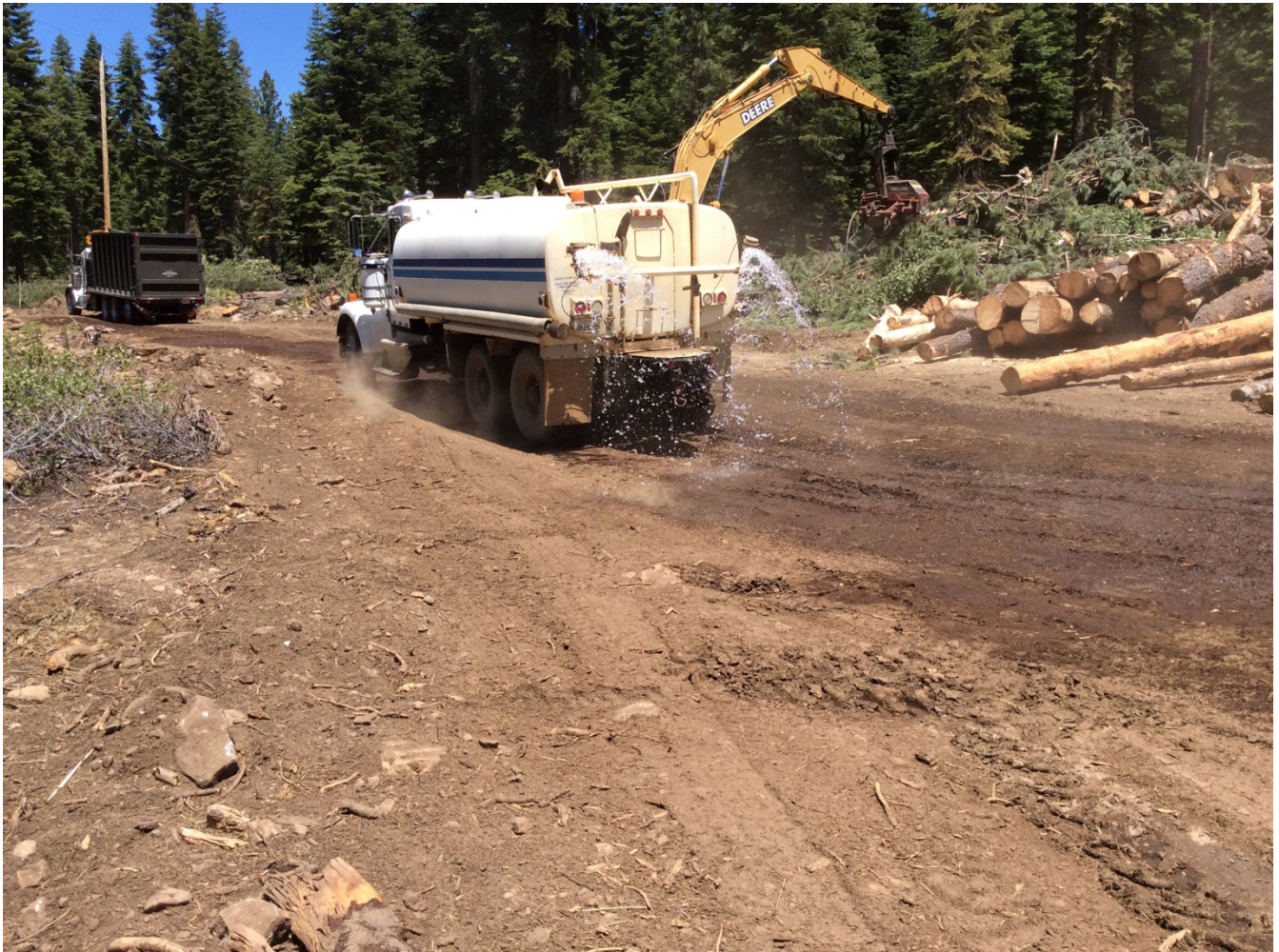
Photo 6: Water truck applying water to control dust at landing near Pole 291169 (APM-AQ-2).
