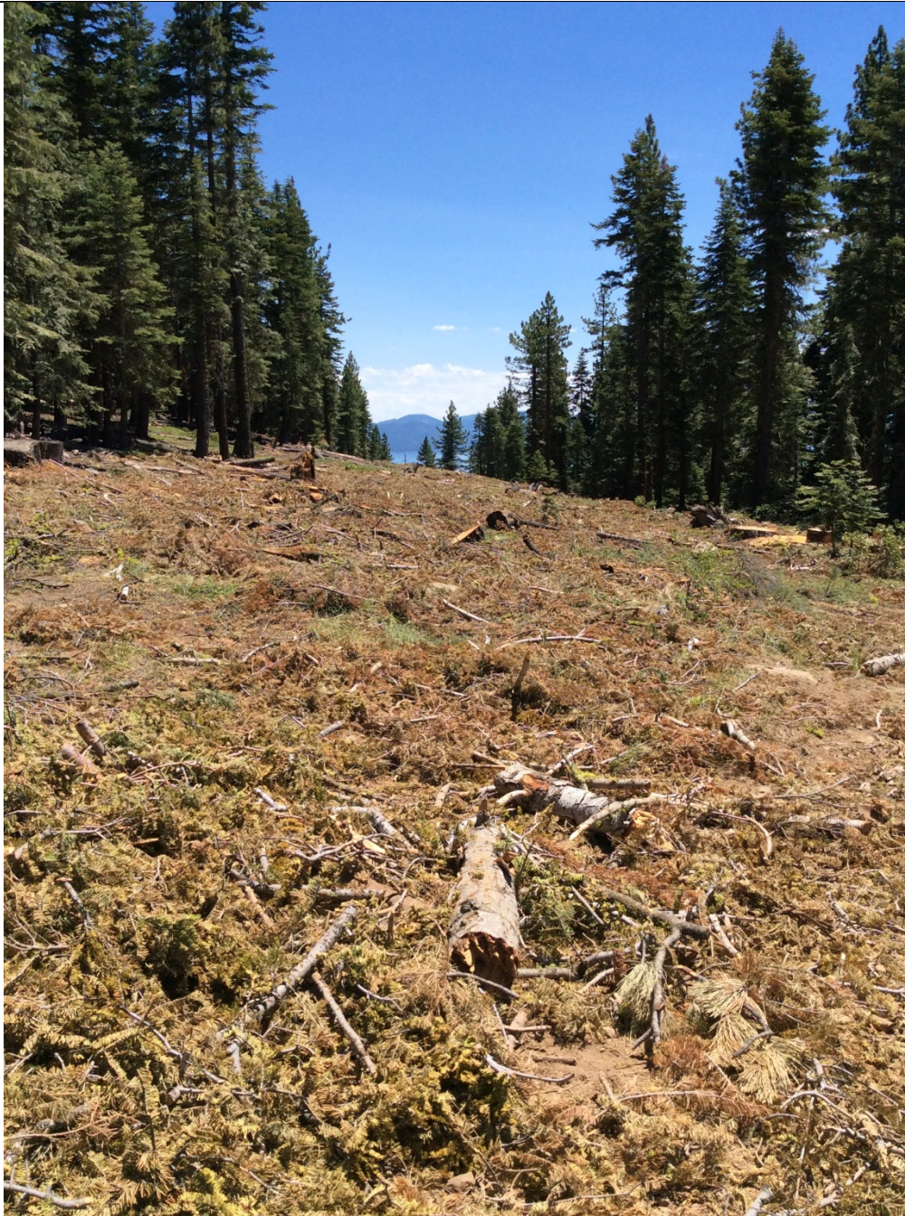
Photo 3: ROW following tree removal and helicopter yarding on USFS property, near Pole 291170. Slash lopped and scattered (APM-SCE-1).
