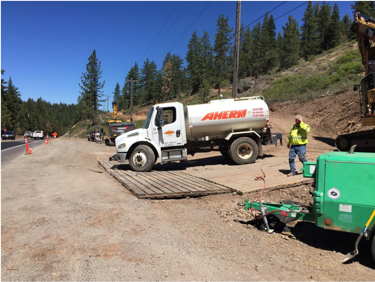
Photo 4: Access road with timber stabilization, compressor for weed cleaning, and water truck to control fugitive dust, near Pole 291129.
