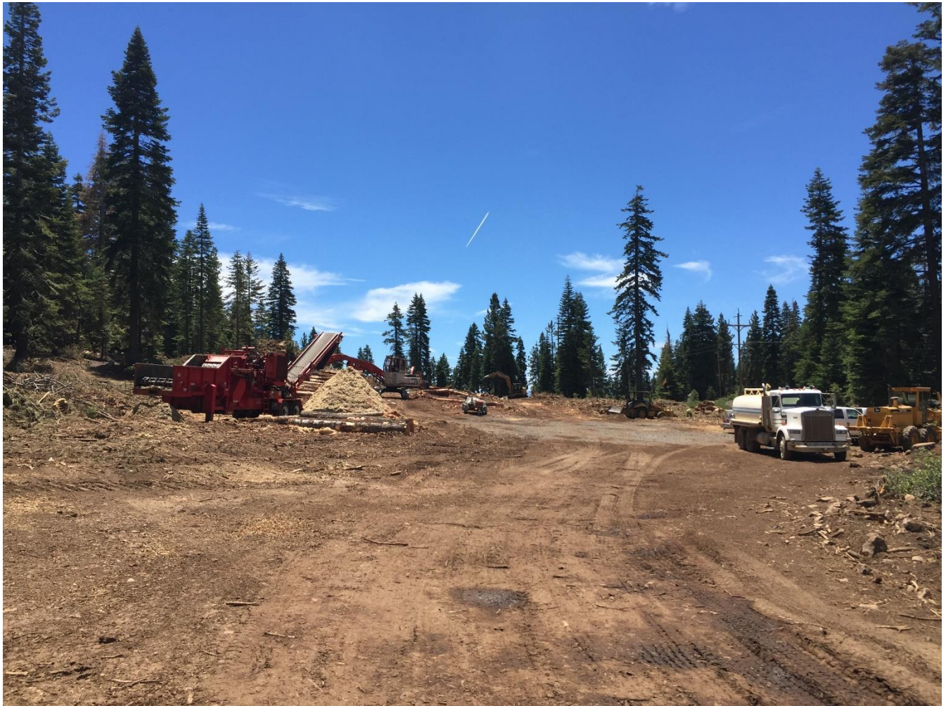
Photo 2: Unit 5 landing (helicopter landing) being cleared and debris chipped preparing for pole installation, near Pole 291169.
