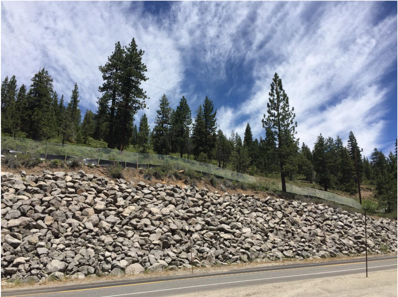
Photo 1: Safety catch fence and silt fence installed below access road and above Highway 267 between Poles 291129 and 291137 to prevent material from rolling onto highway.
