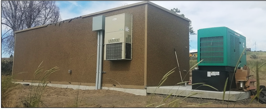
Figure 3-3: Example Regeneration Hut Housing an In-Line Amplifier
