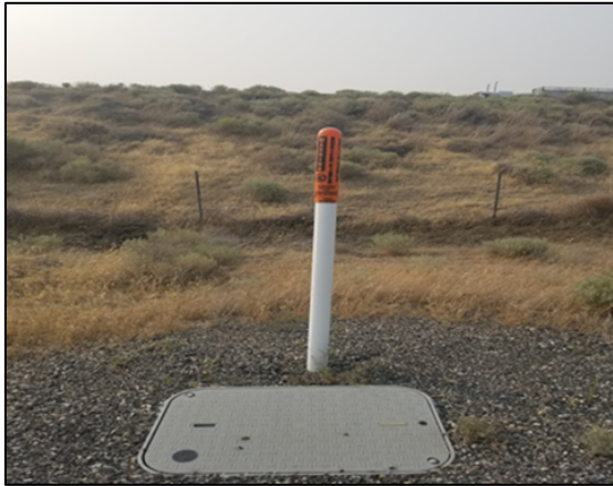
Figure 5.1-6: Example of a Typical Line Marker
