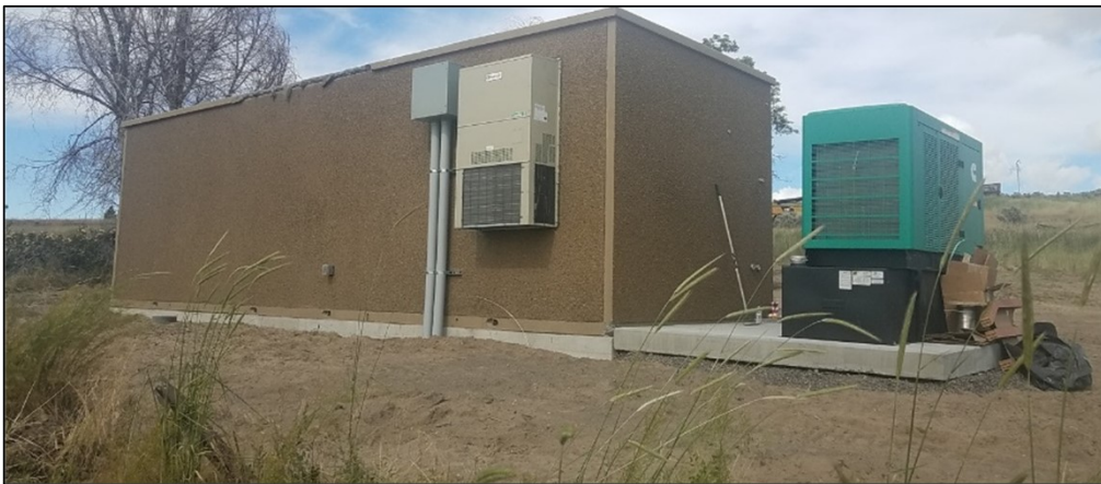
Figure 5.1-5: Example of a Typical Regeneration Hut
