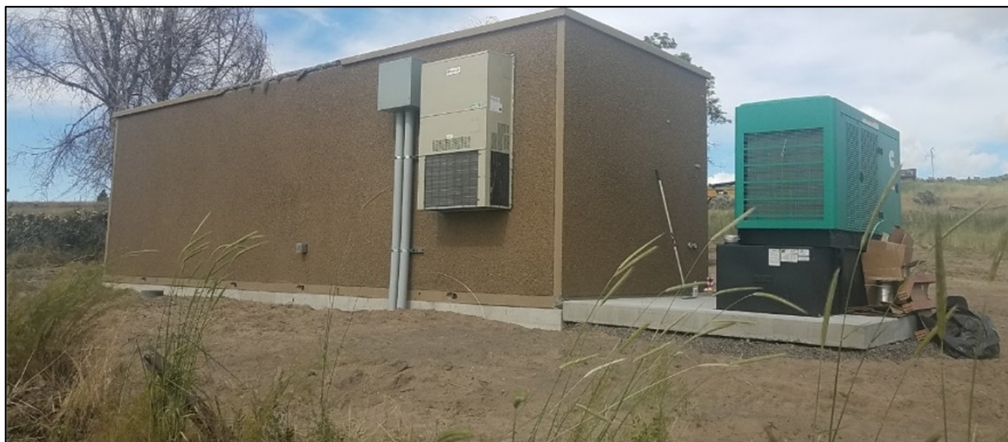
Figure 5.1-65: Example of a Typical Regeneration Hut
