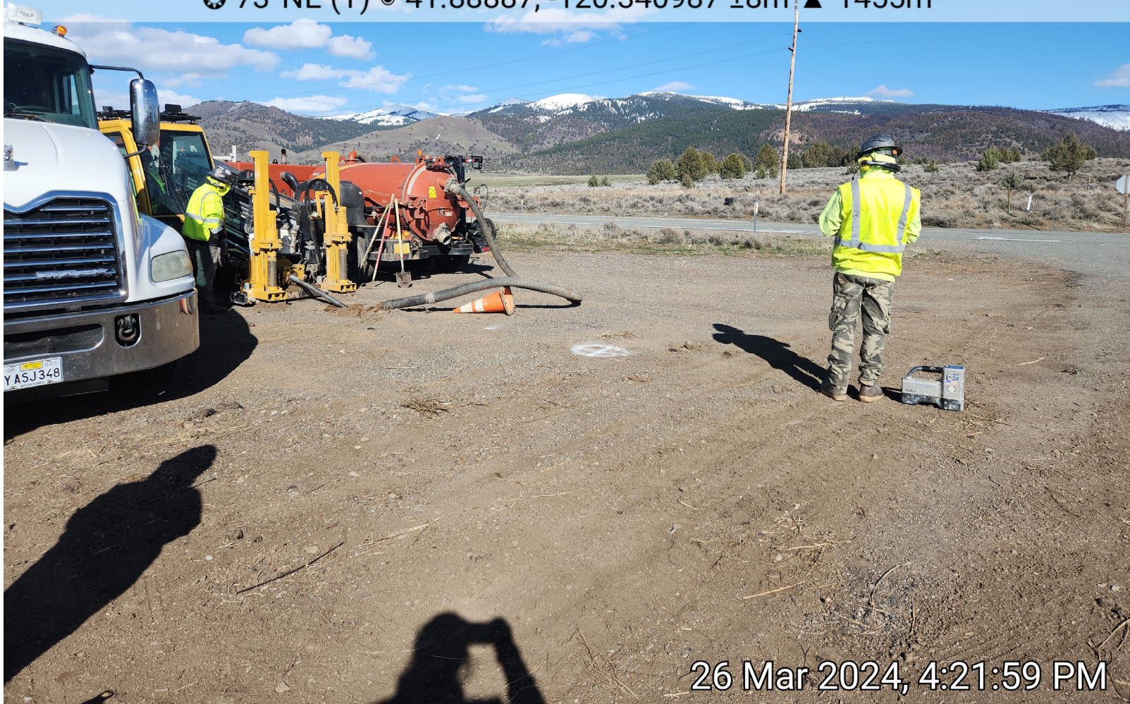
Photo 1: View of HDD at MP 54. The detector to the right shows approximate location of drill
