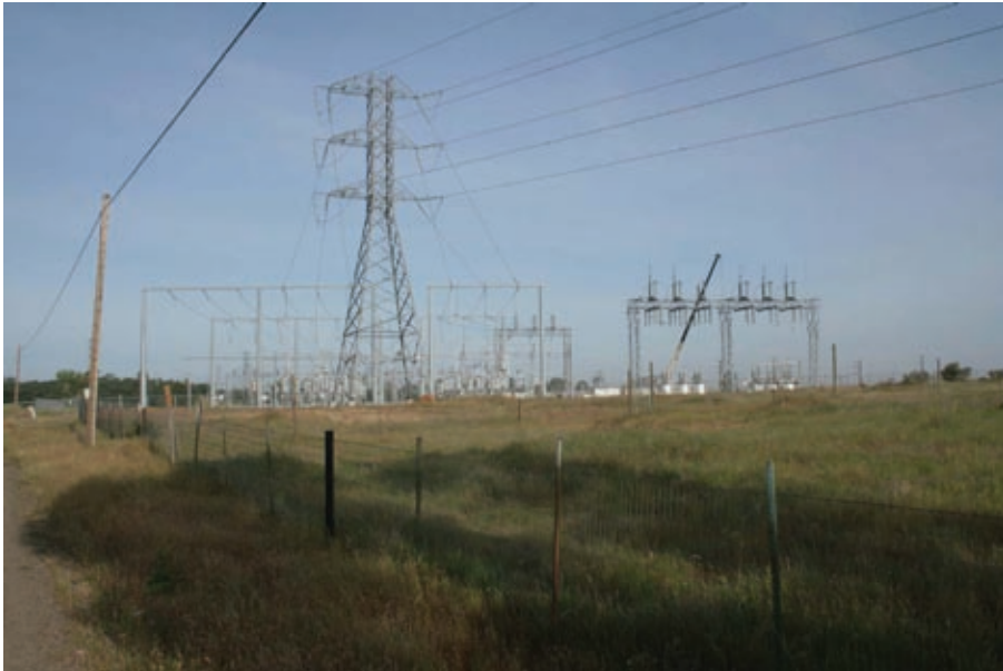
1. Stageline Road looking northwest toward Palermo Substation
