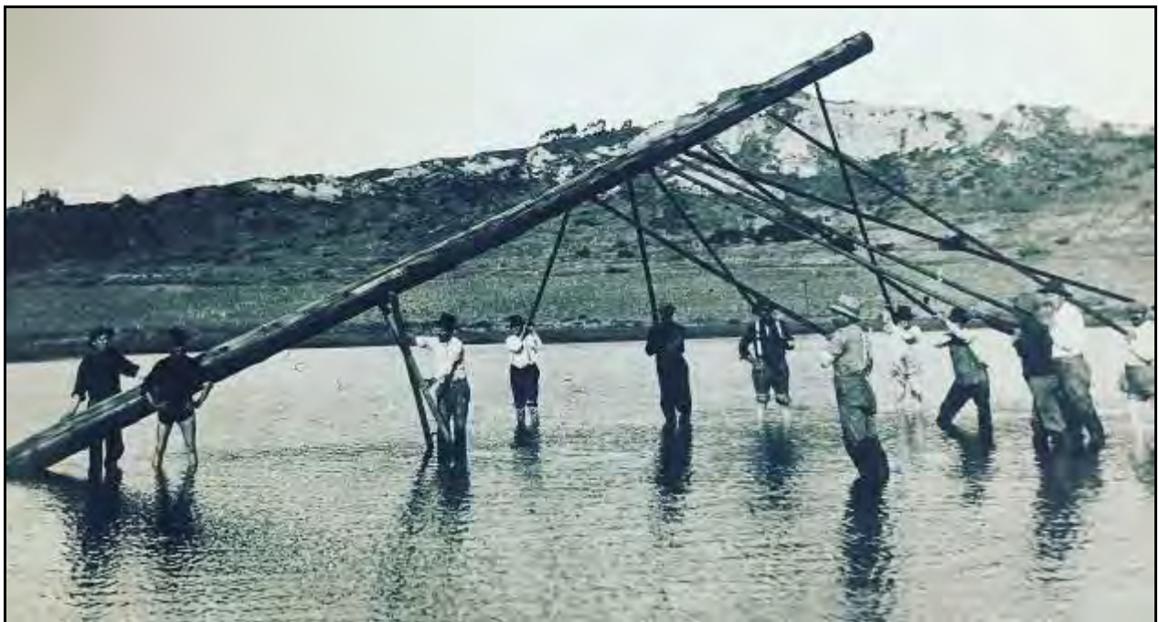
Plate 4. Raising of an SDG&E Pole in San Dieguito Lagoon (Engstrand and Crawford 1991).
