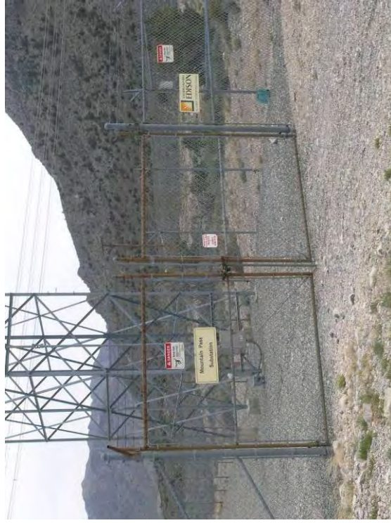
Photograph 15. The existing Mountain Pass Substation. Black cholla is dominant here with scattered piñon and juniper.
