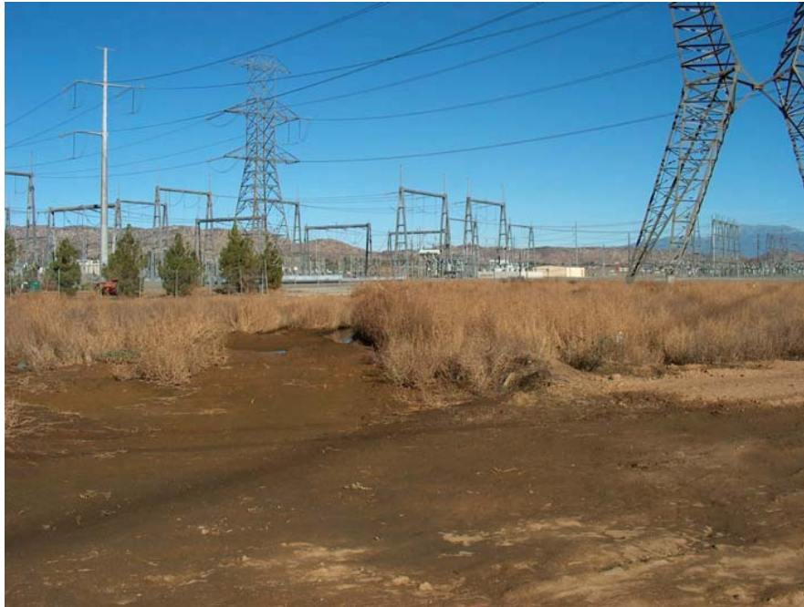
Photo 1. Looking northeast at preferred route's east terminus in the Valley Substation.
