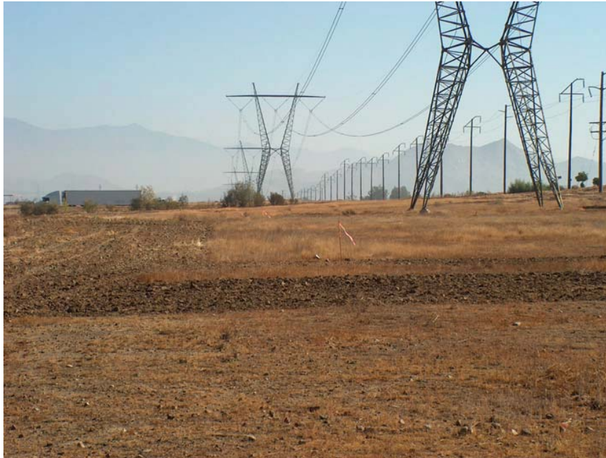
Photo 21. Looking east at the drainage from Photo 20. Truck is on Goetz Road. New alignment will be installed along line of stakes.
