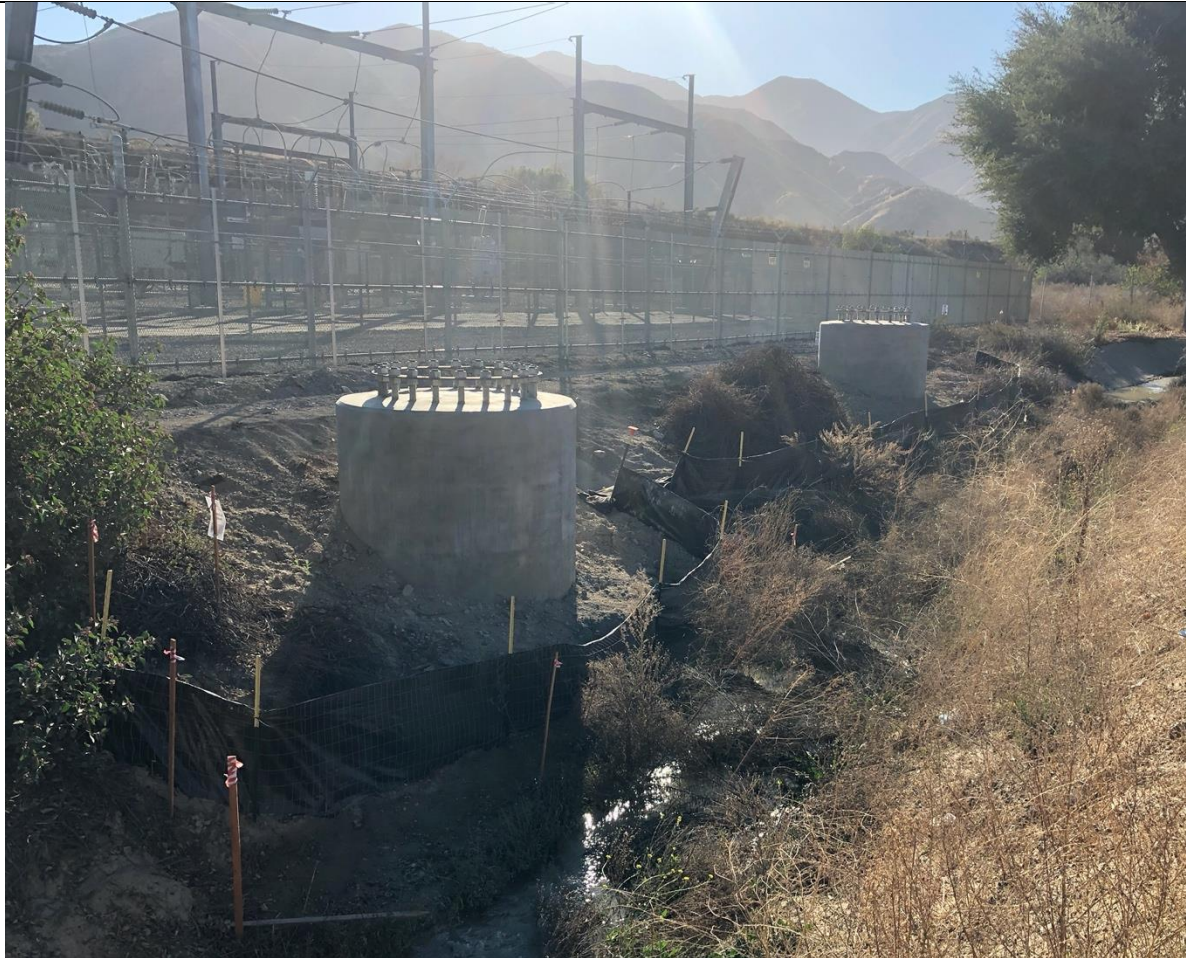
Photo 4 – Newly installed TSSs near the IvyGlen substation. BMPs look good. Photo facing west
