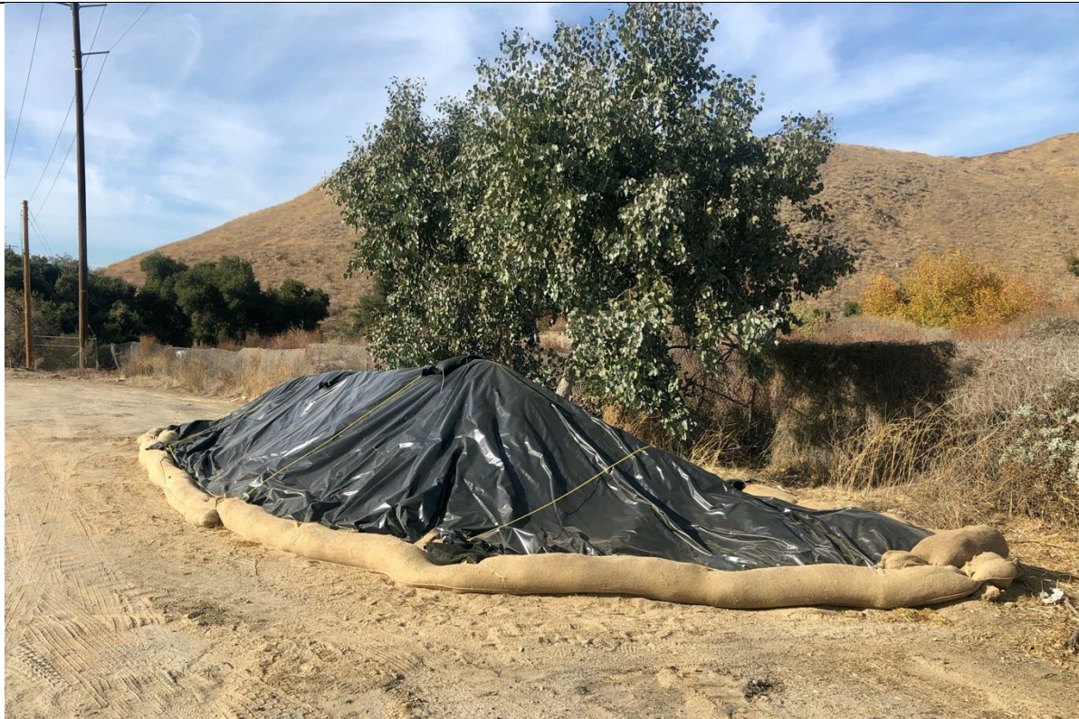
Photo 4 – BMPs over and around a spoil pile. Photo facing northeast
