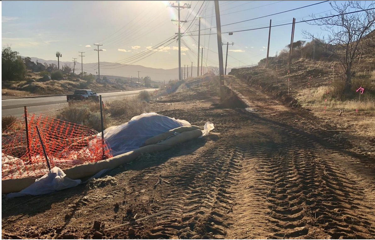
Photo 7 – Road work under the new transmission towers near pole #236. Photo facing west
