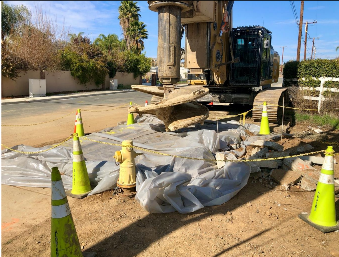
Photo 11 – TSP 313 off of Conrad Rd near HWY 74 has been partially drilled. Crews have shut down for the day and covered the hole. Photo facing east
