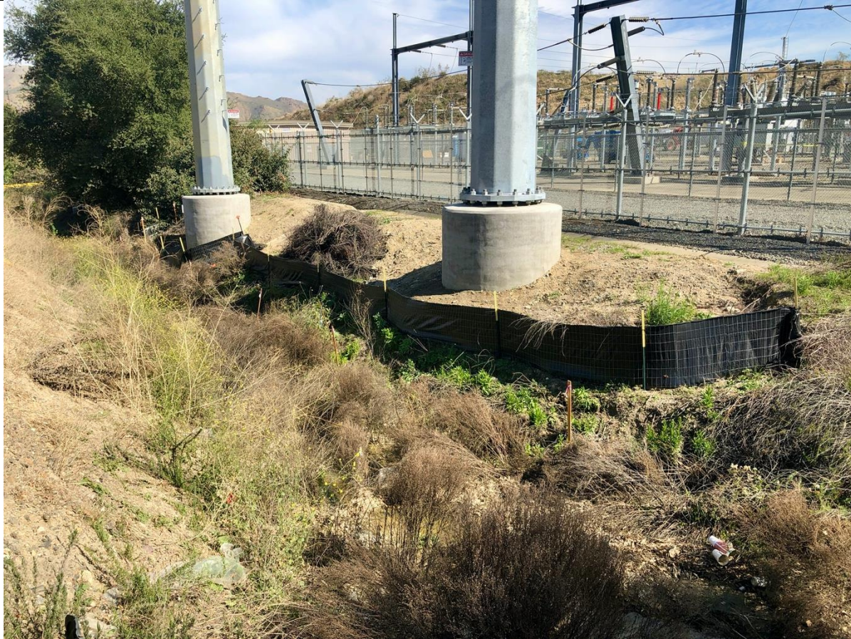
Photo 5 – BMPs remain in place around the TSP foundations in the drainage. Photo facing southeast
