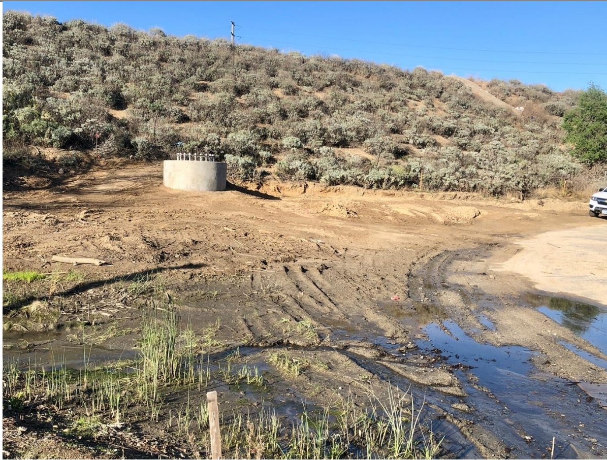
Photo 8 – The area around TSP 520 remains wet from an upstream spring. Photo facing east
