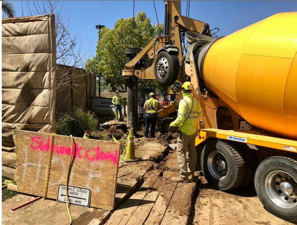
Photo 4 – Pouring slurry in the foundation hole at TSP 358E. Photo facing north
