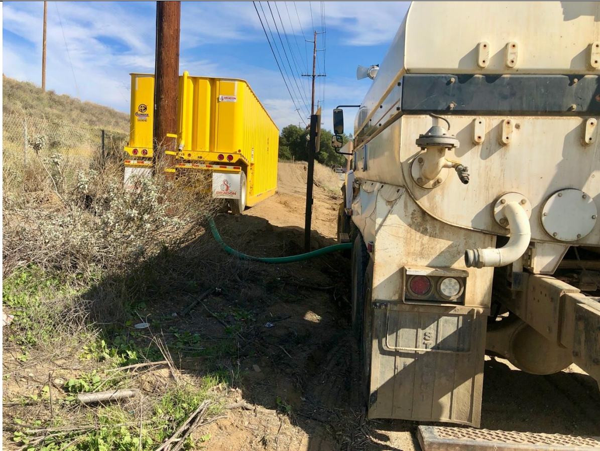
Photo 7 – Baker tanks are in place due to the high water table. Photo facing south
