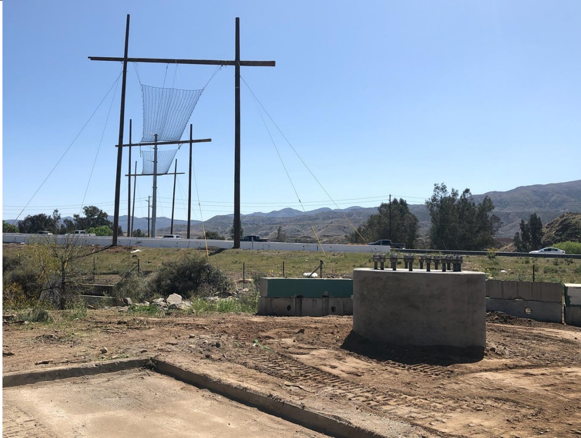
Photo 6 – New foundation at TSP 496-2177E – note the netting for stringing wire over Hwy 15. Photo facing south
