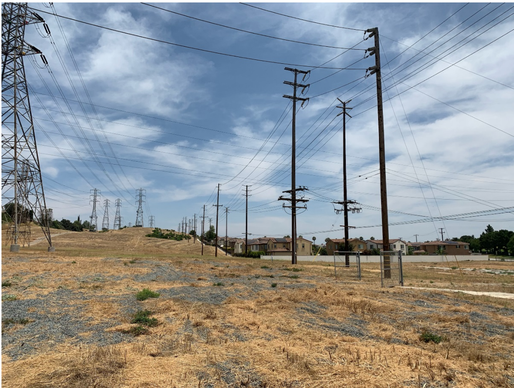
Photo 4. Looking ENE with, from left to right, poles 4017003E, 1551704E, 4017002E, 1551705E, and 4017001E (distant poles and transmission towers not included).
