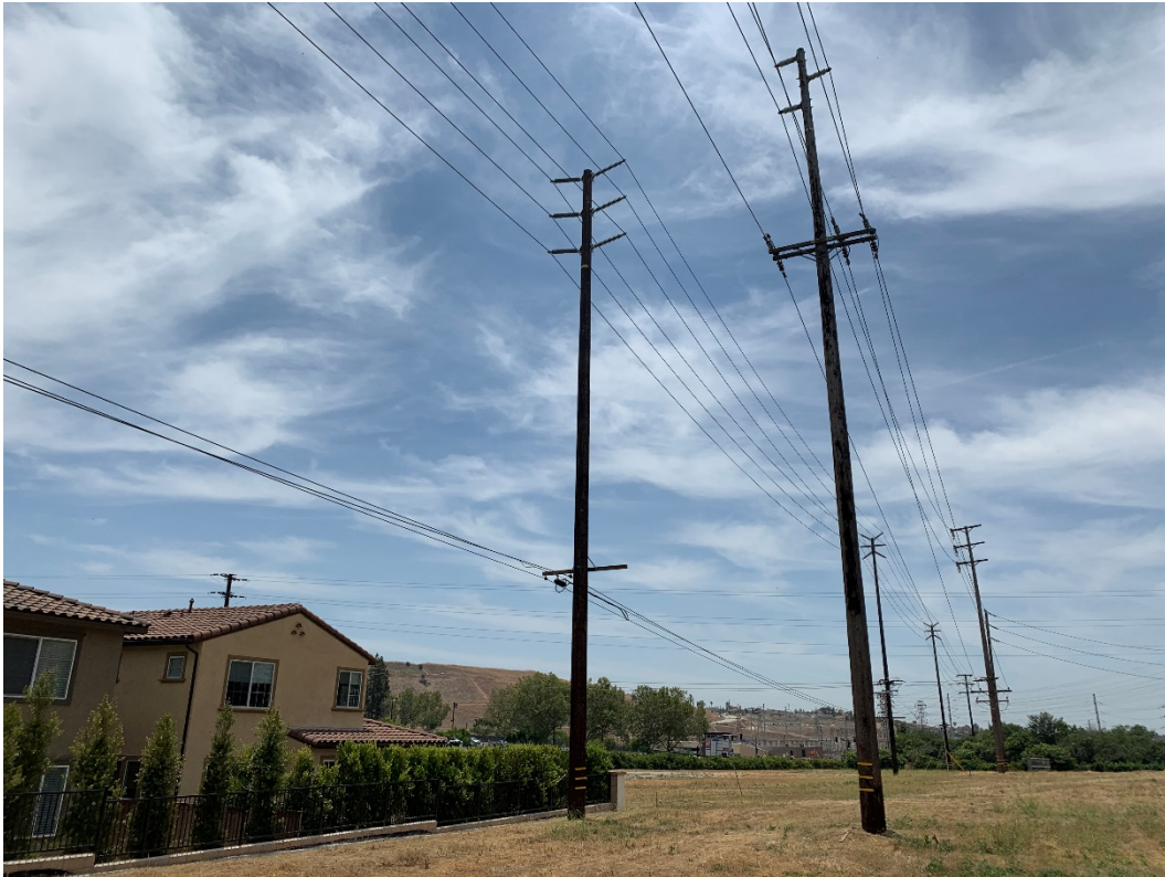
Photo 6. Looking SSW with, from left to right, poles 1551704E, 4017003E, 1551705E 4017001E, and 4017002E (distant poles and transmission towers not included).
