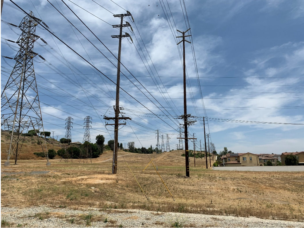
Photo 3. Looking NNE with, from left to right, poles 4017002E, 1551705E, and 1551704E (distant poles and transmission towers not included).
