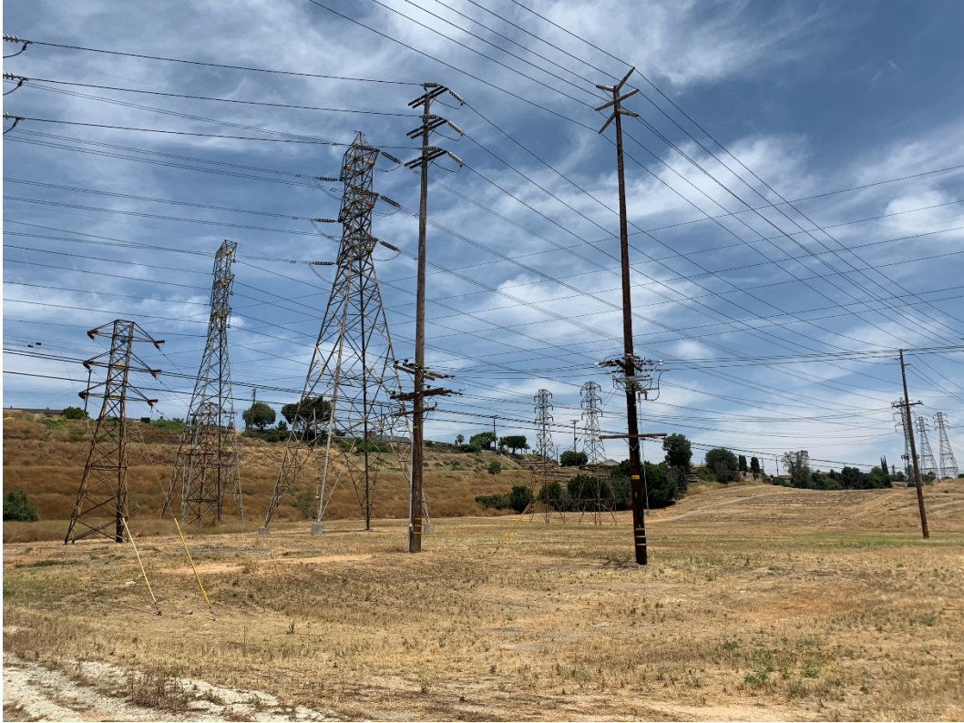
Photo 1. Looking north with, from left to right, poles 4017002E, 1551705E, and 4017003E (transmission towers not included).
