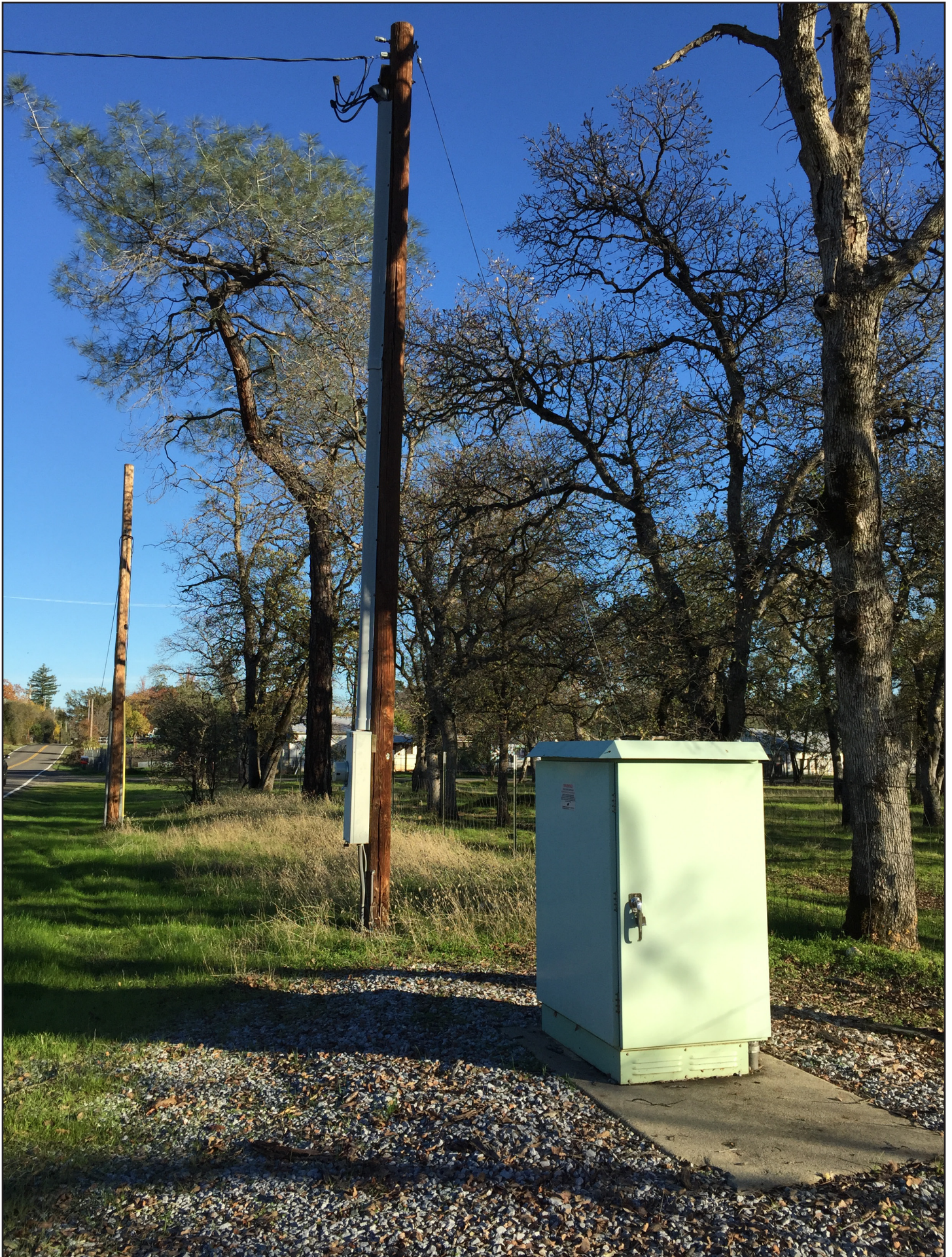
Figure 5.1-2 Existing DLC (equipment cabinet) in Project Area
