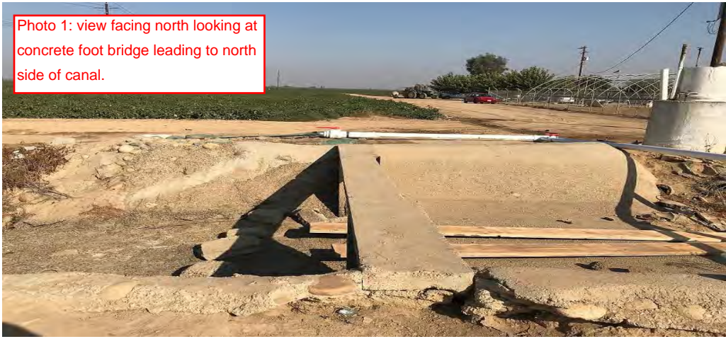
Photo 2: view facing northeast looking at concrete foot bridge and well pump assembly / switch area in background.
