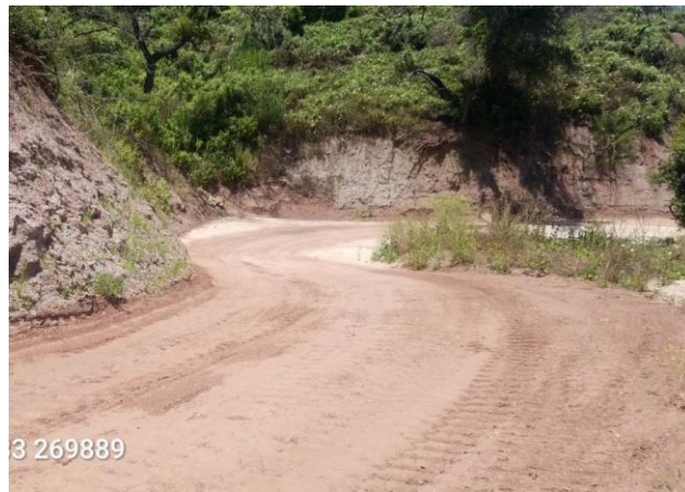
Feature ID: Civil ID 103. Post-construction view of work area at Civil ID 103. Photo taken on July 23, 2019, facing northwest.
