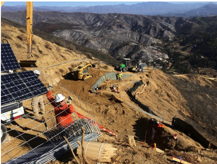
Figure 3. Installation of welded wire walls at Construct 64. Burned areas from the non-project related Thomas Fire shown in the background, December 21, 2017
