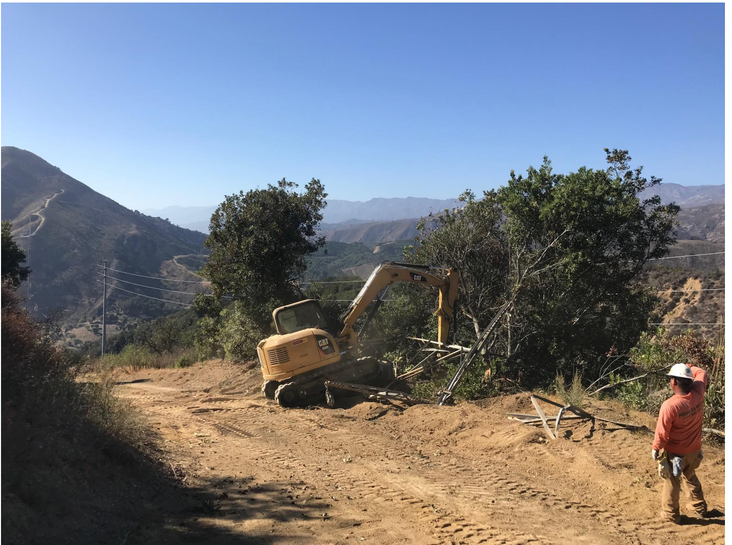
Photo 2: Mini-excavator outside of approved disturbance limits.
