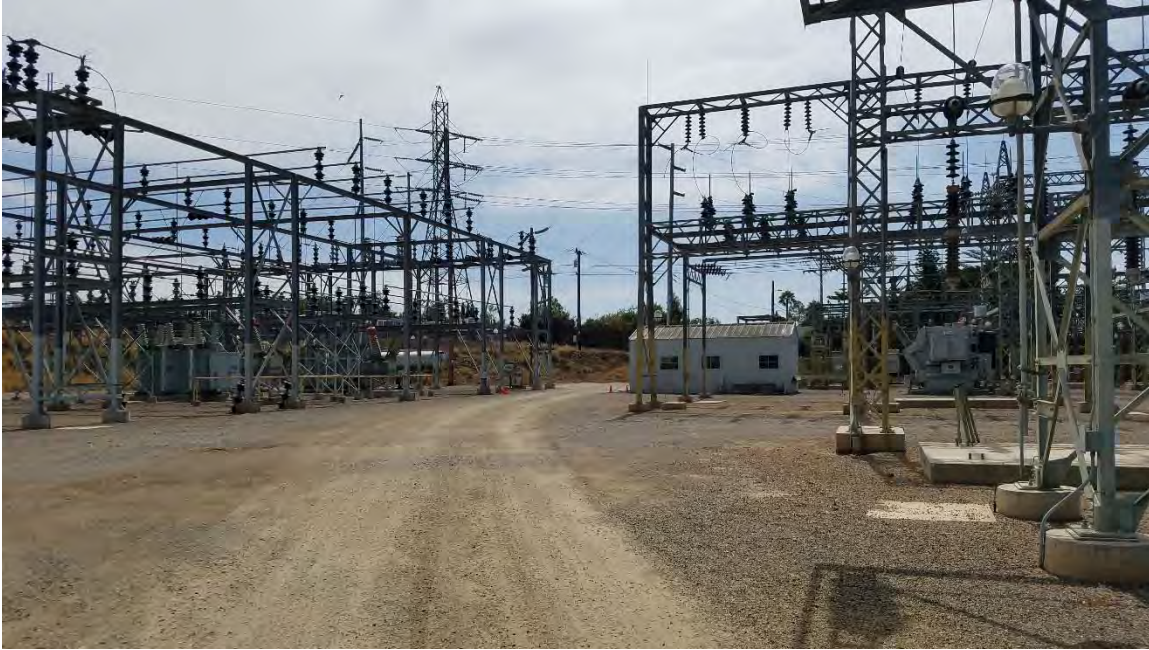
Photo 21. South-facing view into the fenced substation yard; most of the area within the fenced yard is developed, with fountain grass invading the perimeter of the yard.
