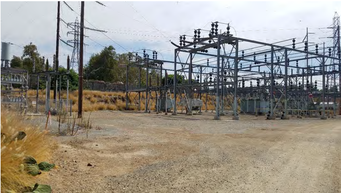
Photo 22. Southeast-facing view of the fenced substation yard.
