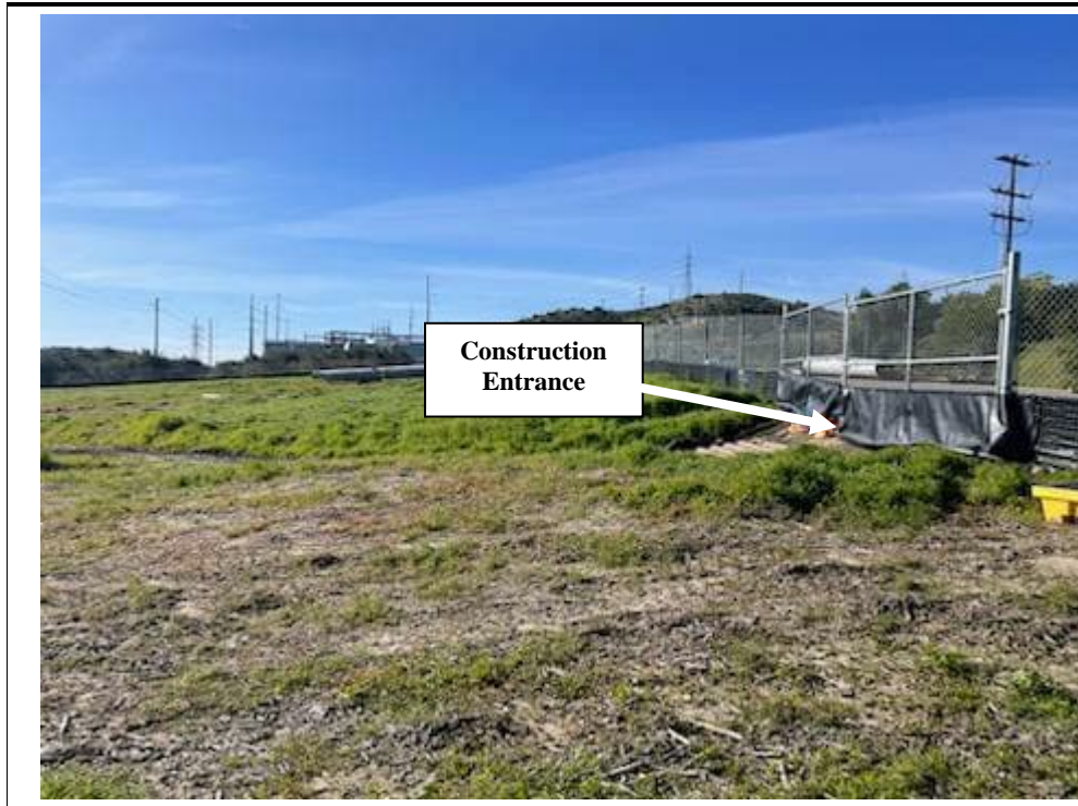
Photograph 1: View of the northwest corner of the MPR-16 staging yard construction entrance, gate, and silt fence BMPs. Facing: South
