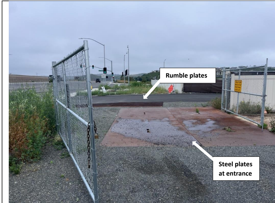
Photograph 1: View of the southwest corner and construction entrance of the Cow Camp Staging Area with previously placed Best Management Practices (BMPs) including rumble plates and flat plates that will be maintained throughout the course of the Project. Facing: Southwest.
