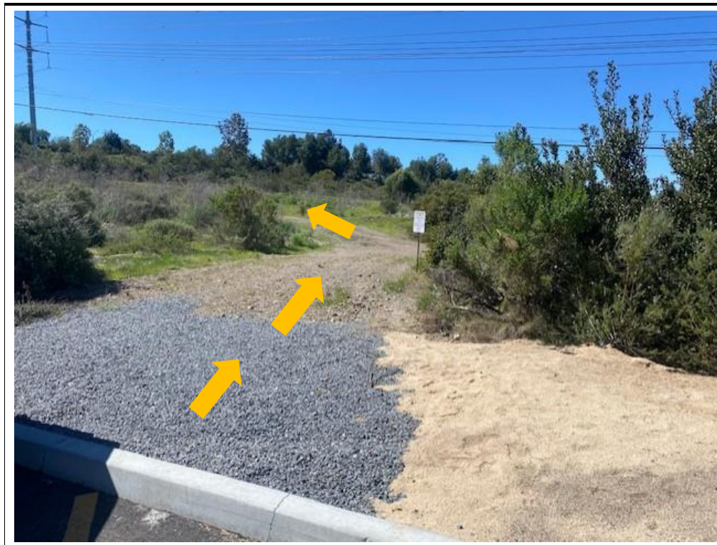
Photograph 6: View of existing SDG&E entrance to the access road that leads to Location 54. The curb will be modified using a wooden ramp. Facing: SW
