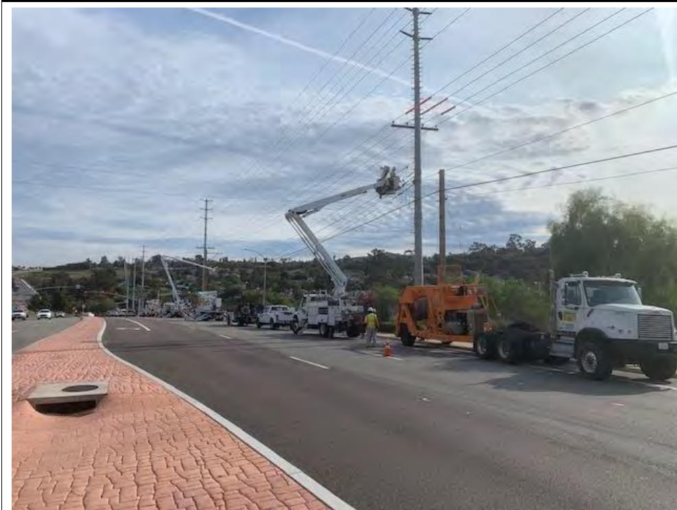
Photograph 40: December 02, 2022. View of OH crews removing old cable at Locations 37 - 42. Facing: East.
