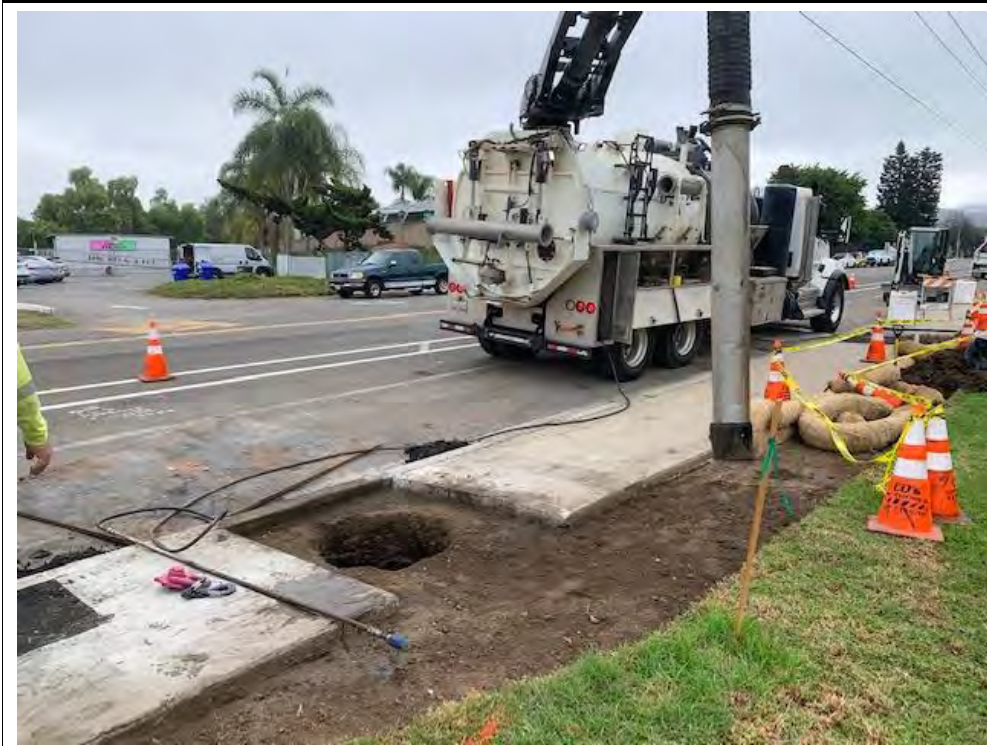
Photograph 4: October 5, 2022. View of crew using a vacuum truck to dig the foundation hole at Location 6. Facing: Southeast.
