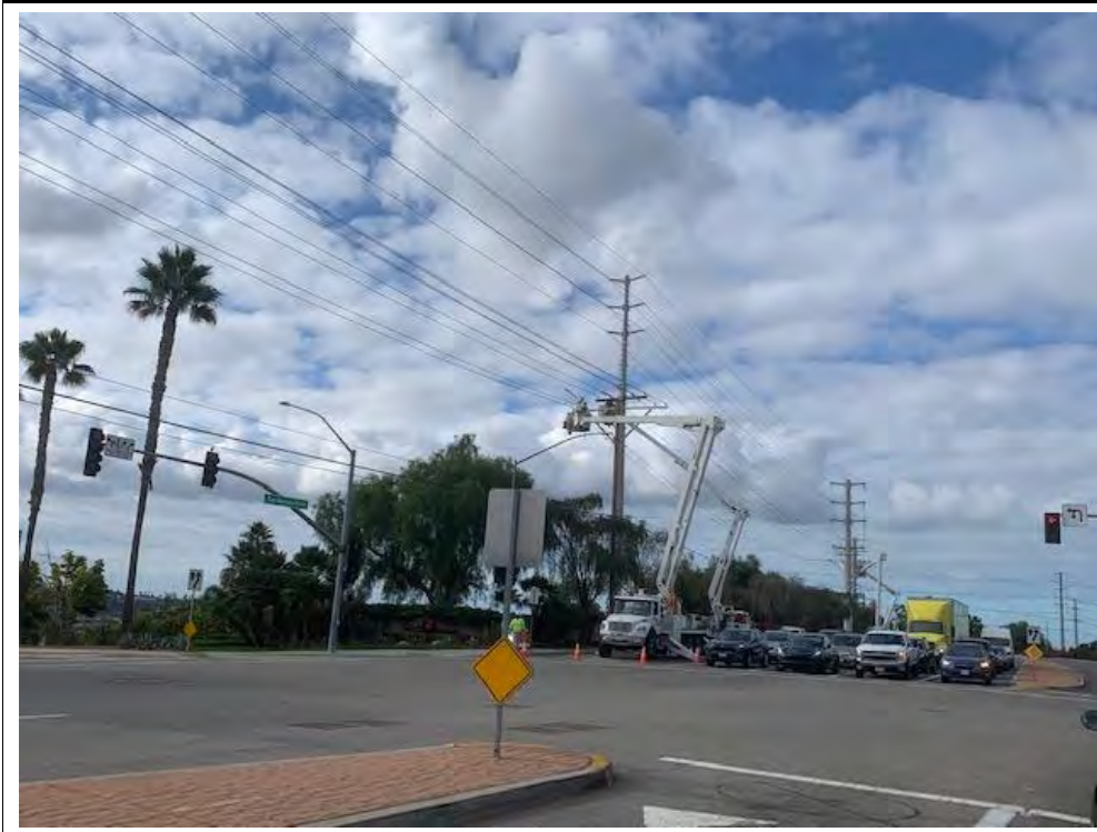
Photograph 44: December 01, 2022. View of OH crews transferring lines over to new pole at Location 47. Facing: West.
