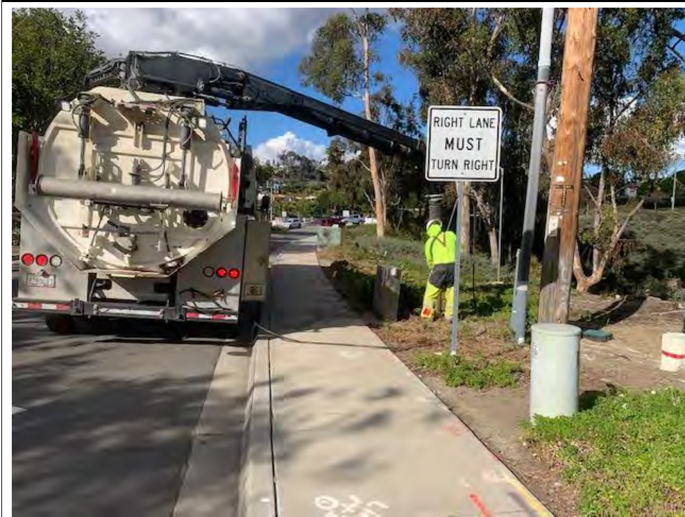
Photograph 46: December 07, 2022. View of crew pot holing for conduit intercept at Location 33. Facing: North.
