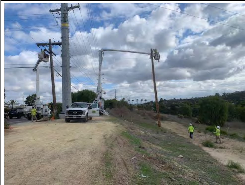
Photograph 42: December 01, 2022. View of OH crews removing old pole at Location 51. Facing: East.
