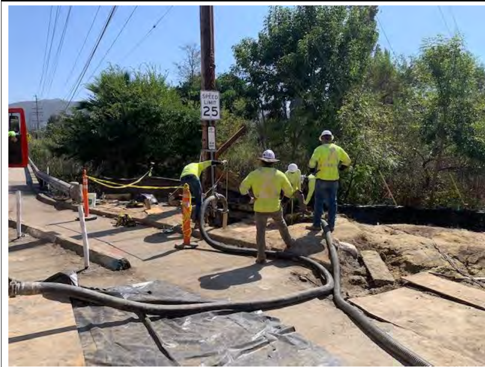
Photograph 6: October 5, 2022. View of crews second day pouring anulus at Location 7. Facing: South.
