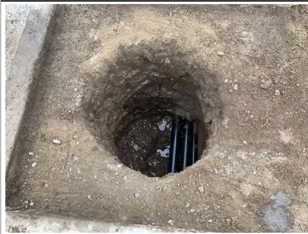
Photograph 5: October 5, 2022. View of multiple conduit lines found in hole at Location 6. Facing: South.
