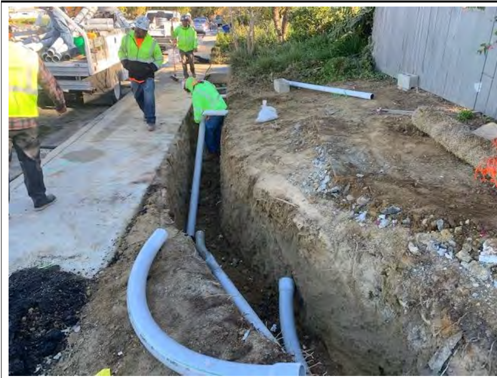
Photograph 39: November 19, 2022. View of OH crews installing conduit for intercept at Location 28. Facing: North.
