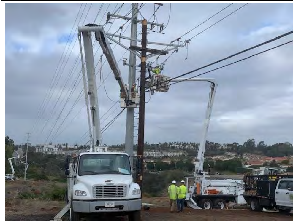
Photograph 45: November 30, 2022. View of OH crews transferring lines to new pole at Location 29. Facing: West.
