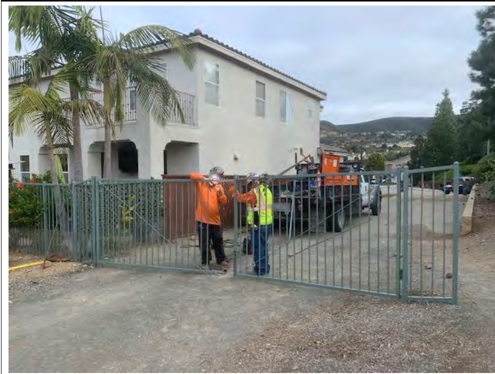
Photograph 41: December 02, 2022. View of crews repairing damaged gate at the entrance to ROW at Copper Court. Facing: East.
