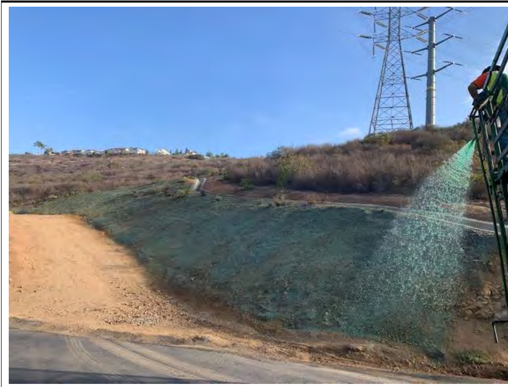
Photograph 25: November 1, 2022. View of crews applying hydroseed to banks at Location 70. Facing: Northeast.
