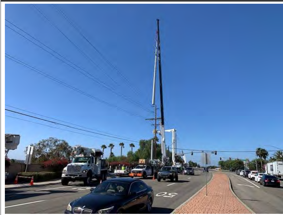
Photograph 23: October 28, 2022. View of OH crews setting pole top at Location 45. Facing: West.
