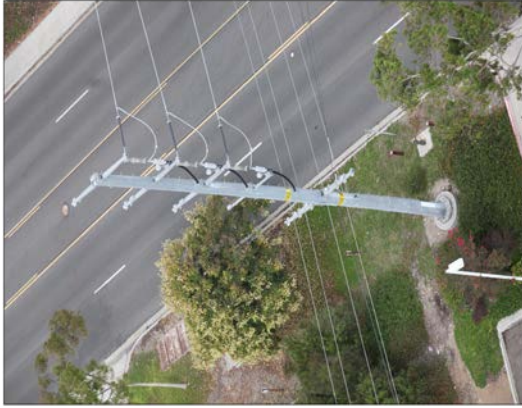
Typical 69kV Double-Circuit Cable Pole with Only 1 Side Installed & Distribution Underbuild
