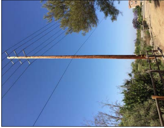
Typical 69kV Double-Circuit Tangent Wood Monopole
