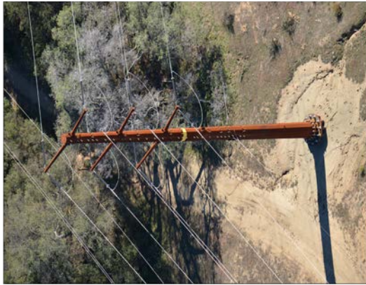
Typical 69kV Double-Circuit Dead-end Weathering Steel Tubular Pole
