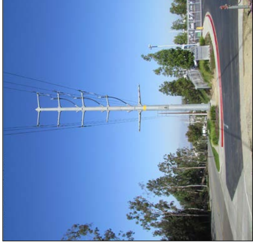
Typical 69kV Double-Circuit Steel Cable Pole with Only 1 Side Installed and 1 Side Pass Through
