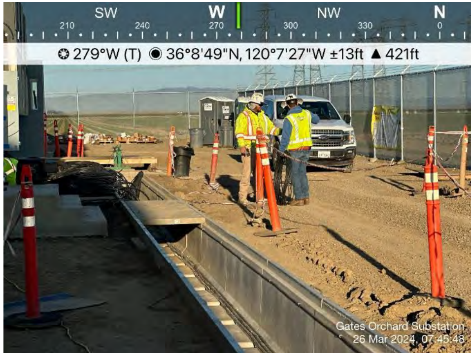
Photo 33. View of crews installing cable in cable trays on north side of enclosure #2. Direction: West. Date: 3/26/2024
