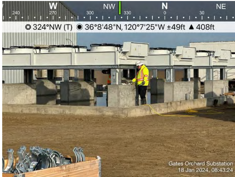
Photo 5. View of crews setting and epoxying anchor bolts for outdoor coolers. Direction: Northwest. Date: 1/18/2024
