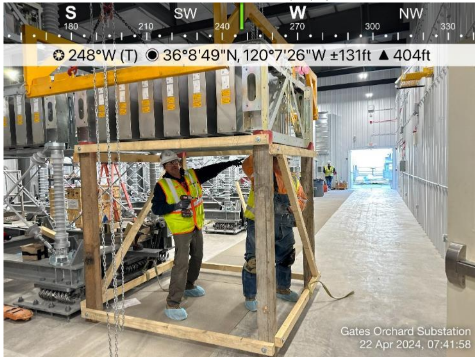
Photo 6. View of compensator installation in enclosure #1. Direction: West. Date: 4/22/2024
