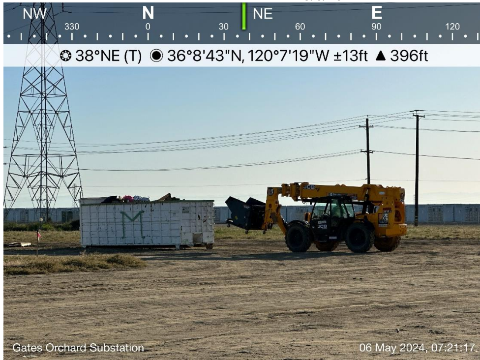
Photo 12. View of lift dumping trash into dumpster. Direction: Northeast. Date: 5/6/2024
