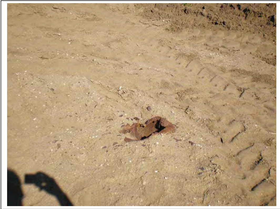
Picture (6). Broken Tip of an Underground Pipe at the Site
