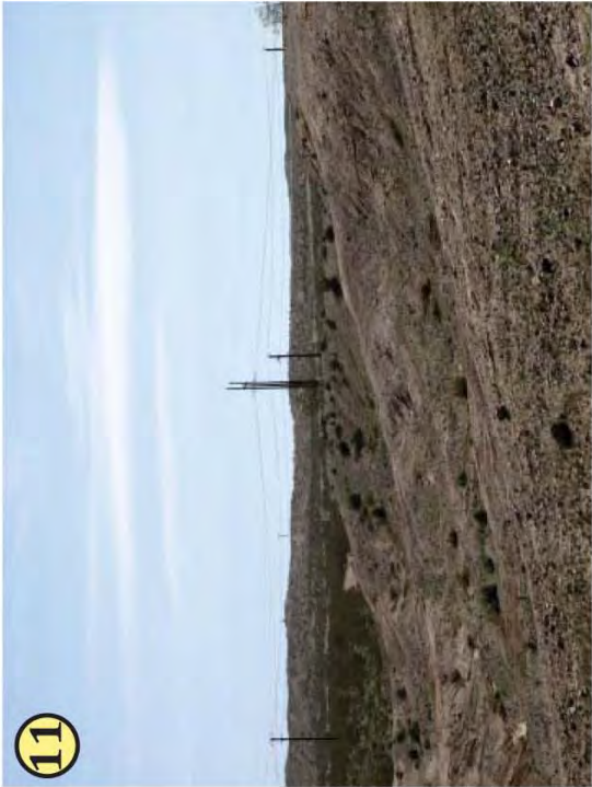
Looking southwest at existing Kramer - Tortilla 115 kV line.
