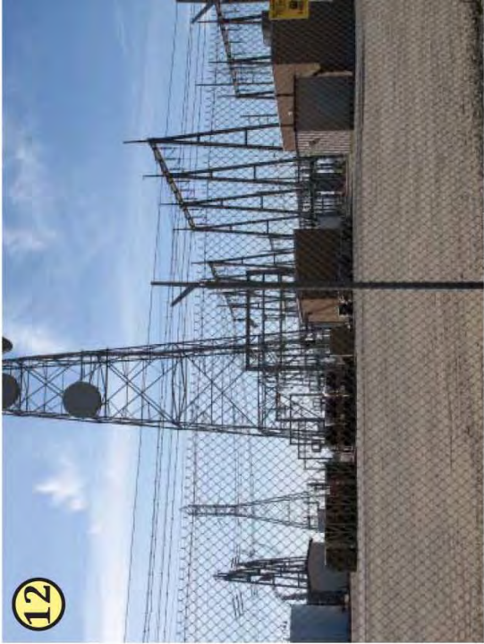
View of Kramer Substation.
