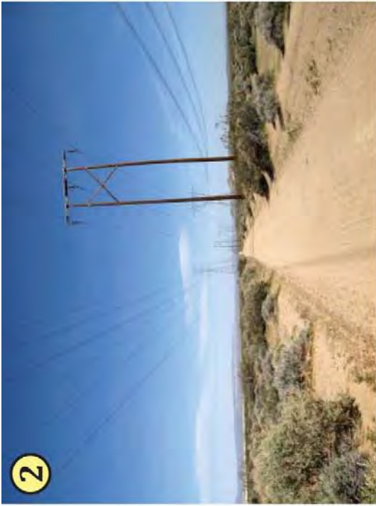
Looking west from Lockhart Substation where new overhead poles are proposed.
