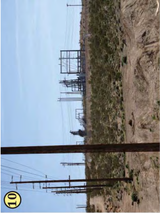
Looking south toward Tortilla Substation.
