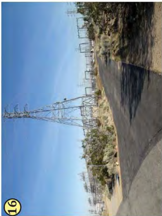
16 View of Victor Substation.
