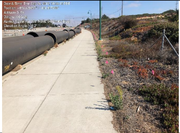
Photo 2. Pipeline storage along General Jim Moore Blvd. Sensitive habitats and plants marked with pin flags
