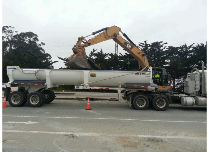
Looking west at Garney excavating trench for waterline main within General Jim Moore Rd.
