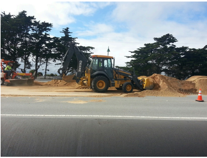
Looking west at backhoe picking up spoil to backfill trench. Sweeper used to clean road.
