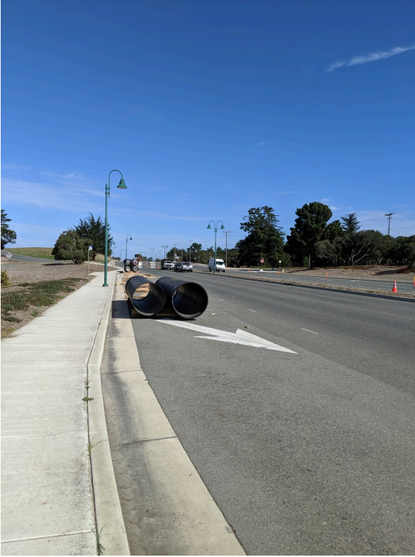
Pipes being stored on Army land on SB GJM by the Bayonet Golf Course.
