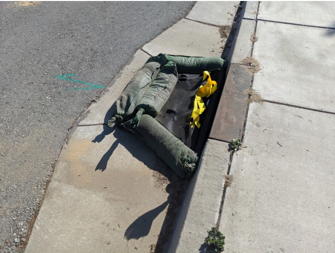
filter fabric and gravel bags over stormwater drains along general Jim Moore
