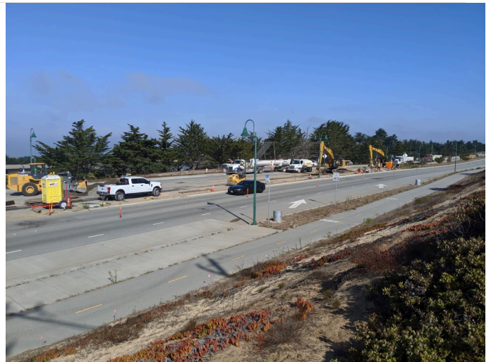
view of work area and soil deposition truck using dust cover, facing NW
