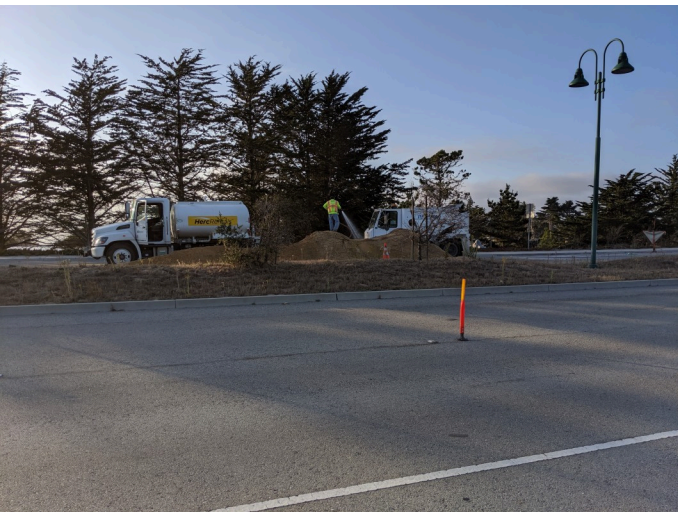
dust mitigation on active soil storage on general Jim Moore, facing W
