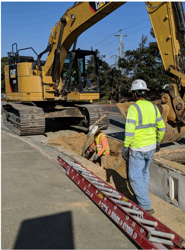
Abandoned conduit line was discovered at about STA 0+35
