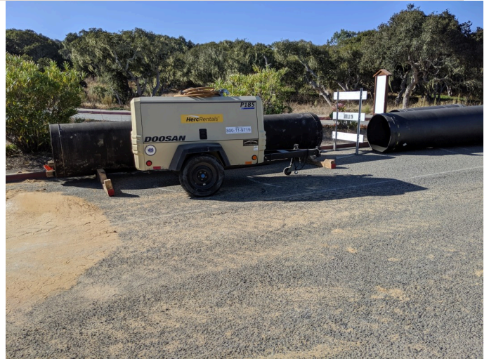
relocated generator, facing SE
