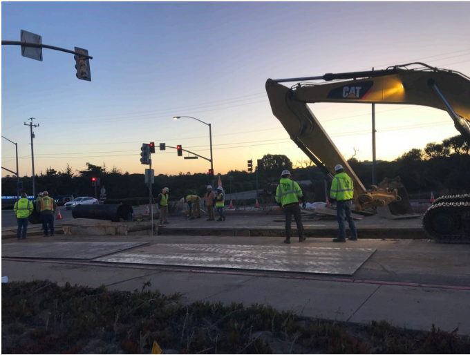
pipeline installation at the intersection of light fighter and General Jim Moore
