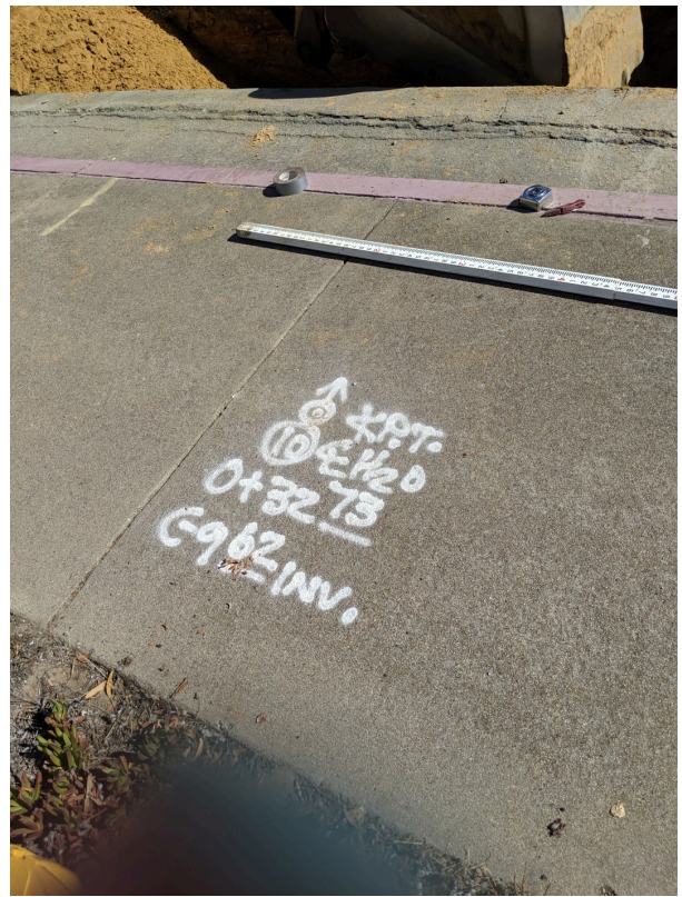
Utility location was different at the field than shown on plans
