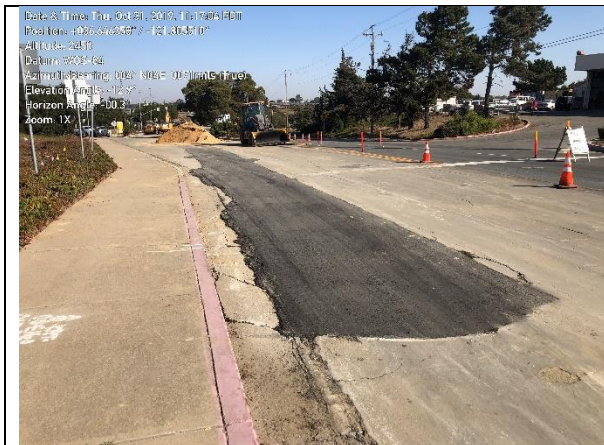
Photo 1. Completed pipeline installation in first section north of Army lands on General Jim Moore Blvd.
