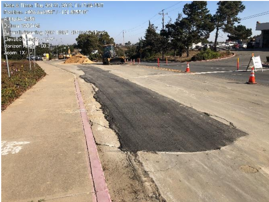
Photo 1. Completed pipeline installation in first section north of Army lands on General Jim Moore Blvd.
