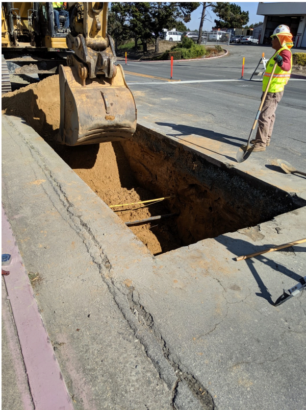
Gas line that was at STA 0+32 but shown at STA 0+20 on plans
