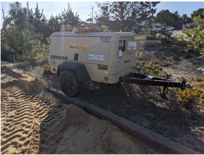
generator outside of work area facing S
