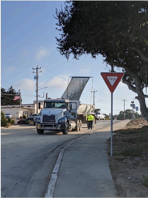
dust mitigation over soil transport truck, facing S on Gen Jim Moore
