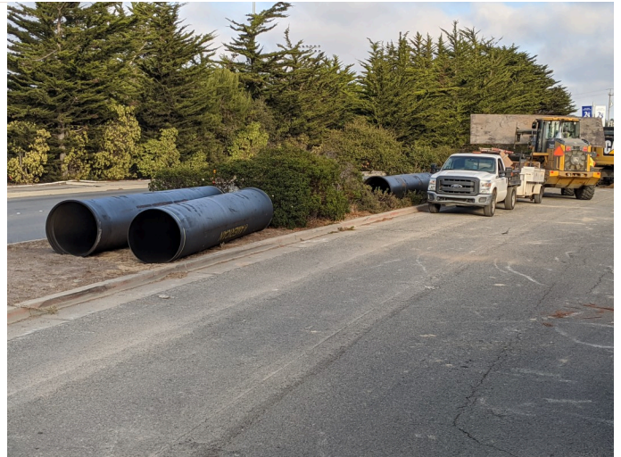
pipeline being stored outside of project area in median on Lightfighter ave, facing E
