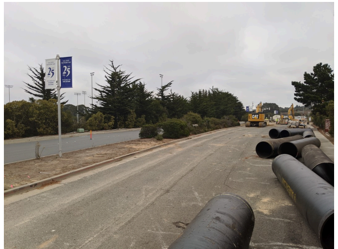
pipeline removed from unapproved storage area on Lightfighter, facing E
