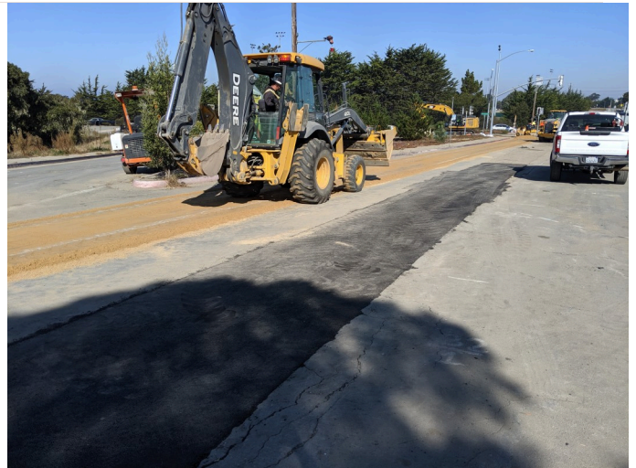
sand absorbing of spilled hydraulic fluid in isolated roadway, facing E
