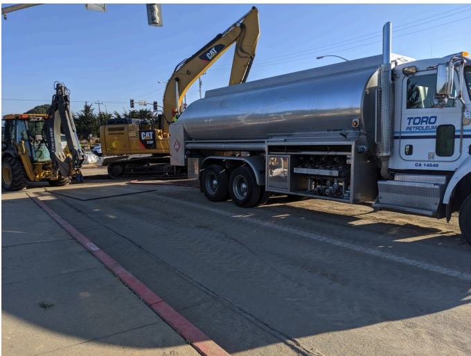
fueling of equipment in roadway away from storm water drains, facing N
