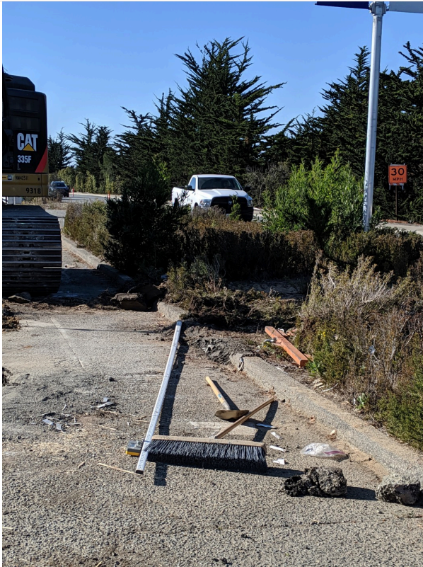
Excavator backed into the median on Lightfighter. Curb and vegetation were affected
