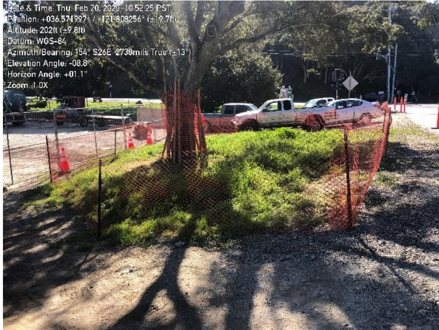
Photo 3. Tree protection installed around coast live oak tree in front of York Road staging area
