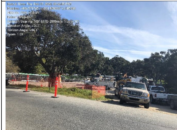
Photo 3. Tree protection being maintained around drip line of oak tree in front of staging area
