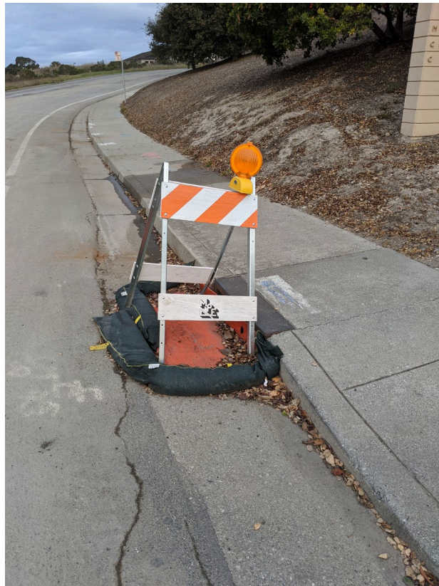
Photo 2. Stormwater drain protection in need of maintenance. (3-9-2020)
