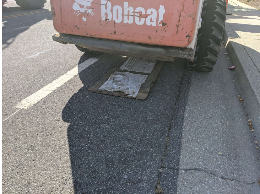
Photo 1. Hazardous spill protection under equipment on alignment. (3-13-2020)
