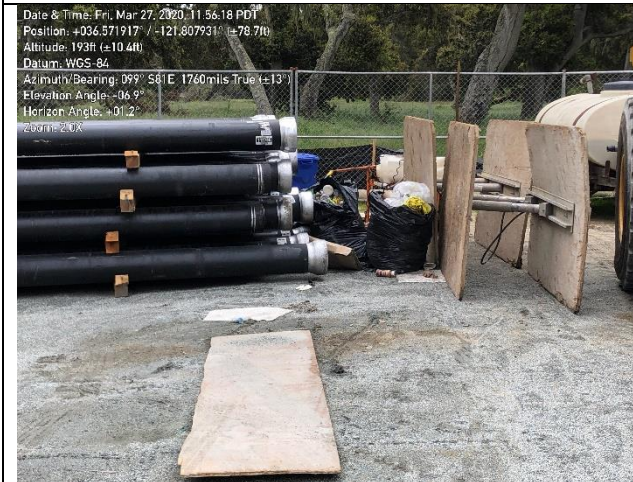
Photo 3. Trash improperly stored within staging area.
