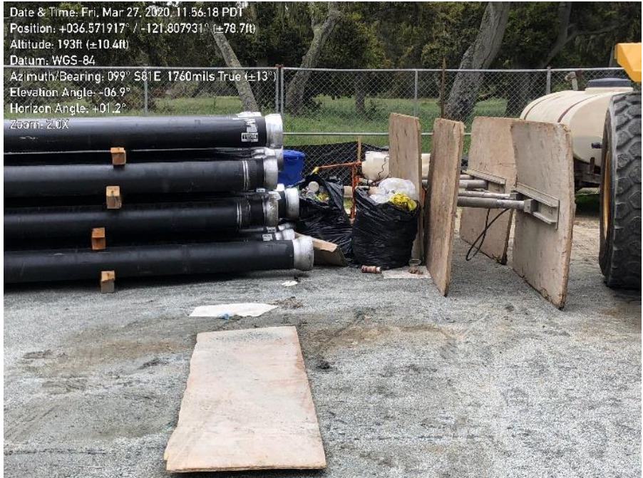
Photo 3. Trash improperly stored within staging area.
